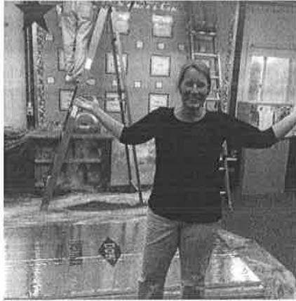
Grade 1 teacher Amy Spivack poses while new insulation is installed in her room.
