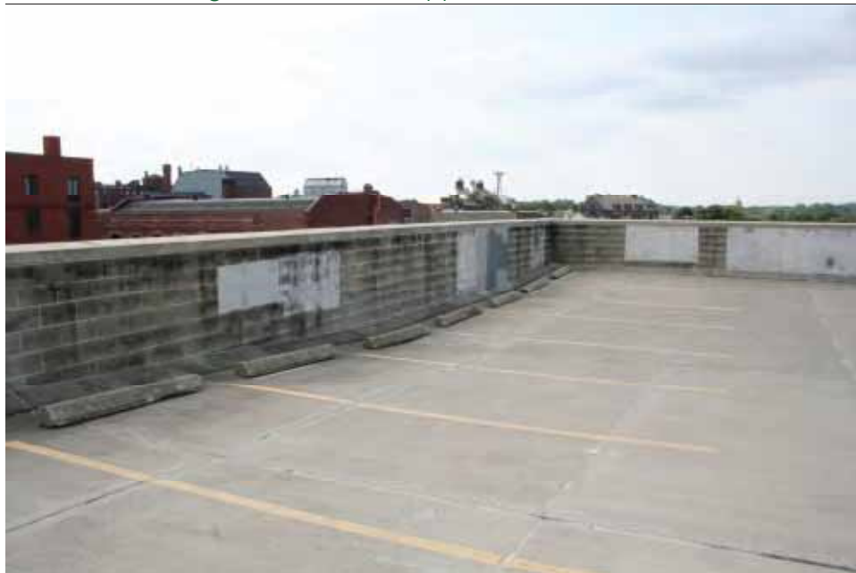
Photo 32 Level 5 – South Elevation. Interior view of CMU wall. Note staining and detractive appearance on wall surface.
