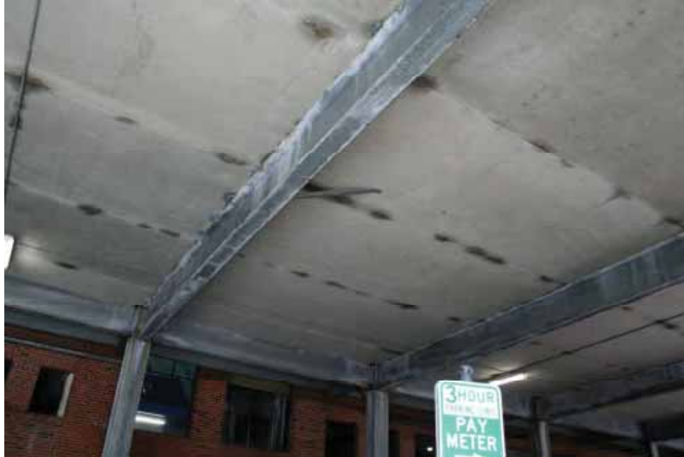
Photo 19 Level 2 – Floor underside expansion area. View shows leakage and staining along filigree plank joint lines.
