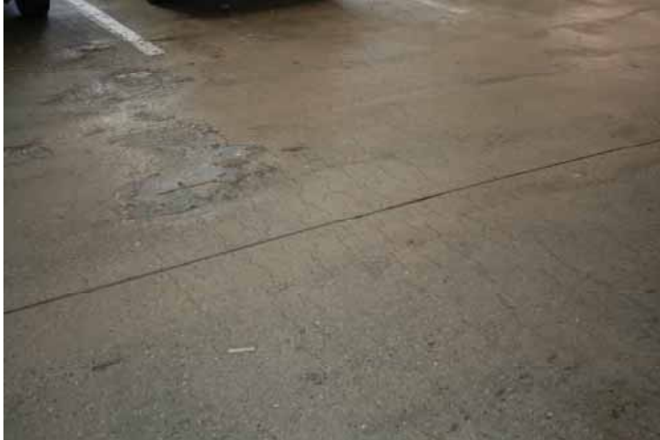
Photo 9 Concrete deterioration (spalling) in flexural crack zone along steel framing.
