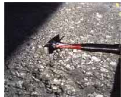
HEAVY SURFACE SCALING
