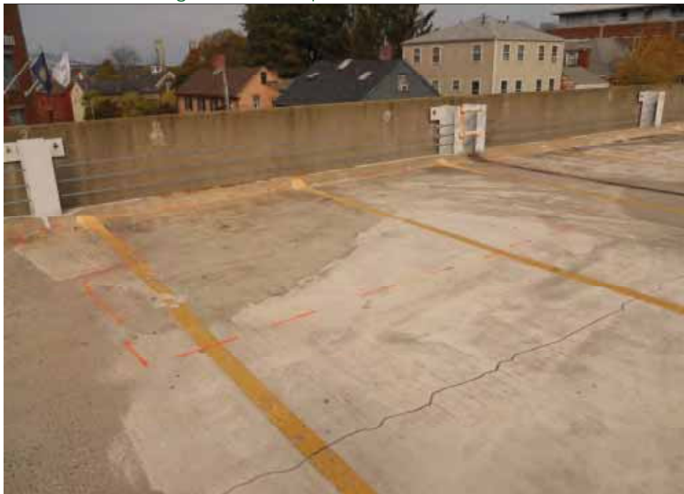
Photo 10 Level 4 – Thinset overlay material applied on floor. Note cracking and bond separation.
