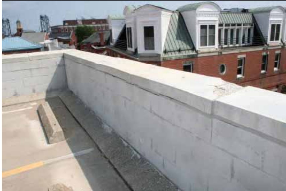
Photo 31 Level 5 South Elevation – South Barrier Wall. Shows capstone deterioration and CMU deterioration. Note missing flashing below capstone.
