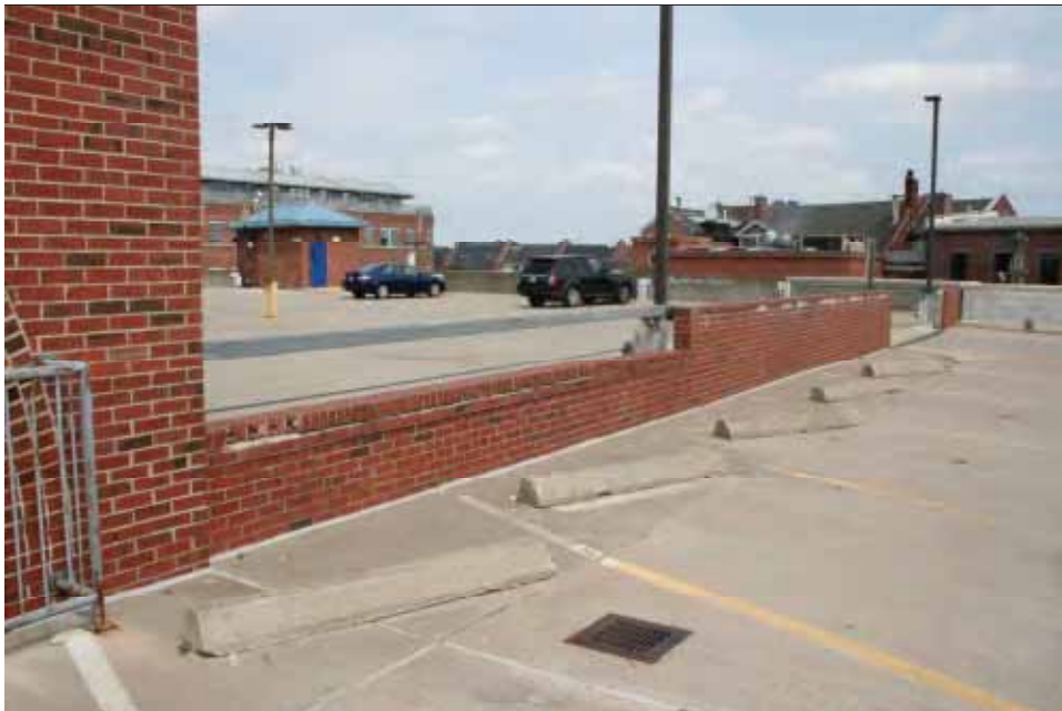
Photo 30 Interior Barrier Wall. View of significant damage and deterioration.
