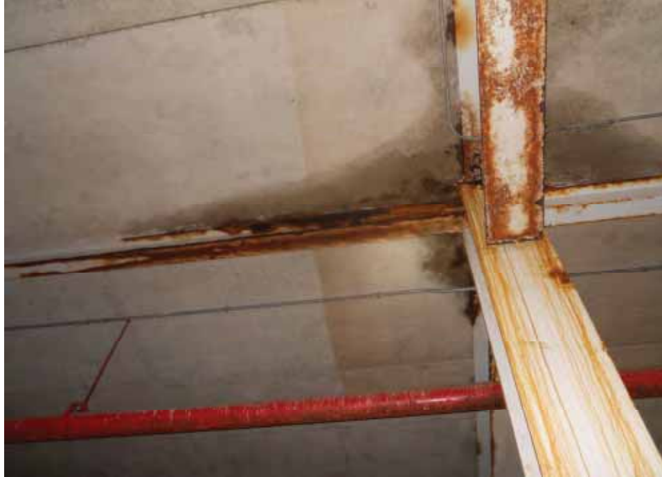
Photo 15 View of moisture saturation and deterioration on filigree planks. Note corrosion on fire protection pipe.
