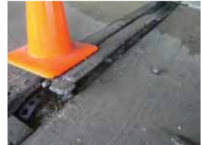
FAILED EXPANSION JOINT
