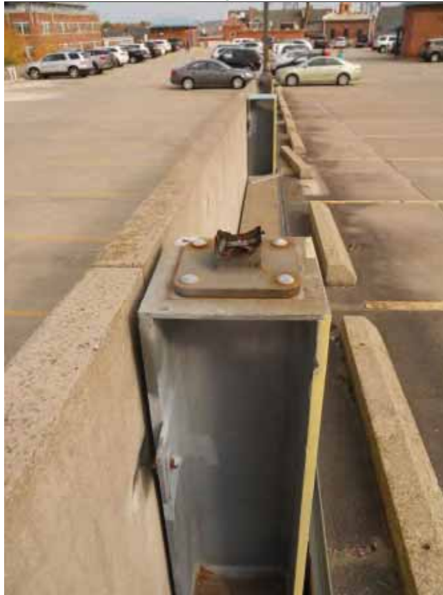
Photo 36 Level 5 – Missing Light Pole. Note corrosion at light pole base.
