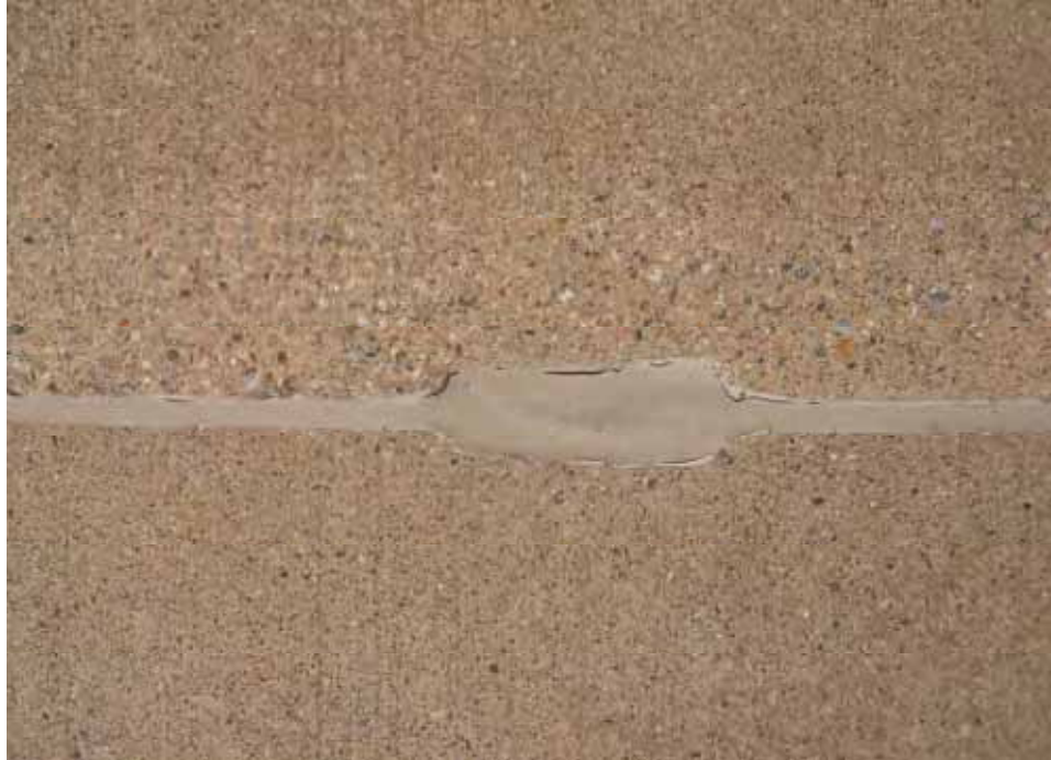
Photo 17 Level 5 – Precast filigree joint sealant with intermittent sealant adhesion failures.
