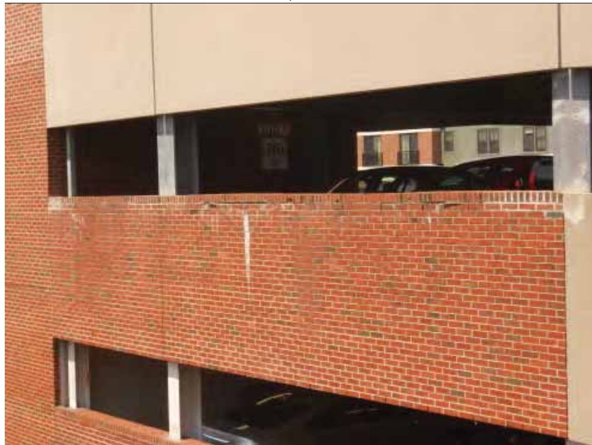
Photo 24 South Elevation. View shows brick masonry deterioration and displacement.
