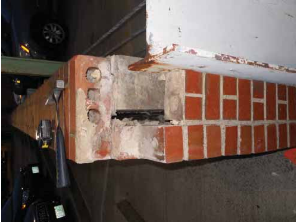
Photo 33 Barrier wall masonry damage.
