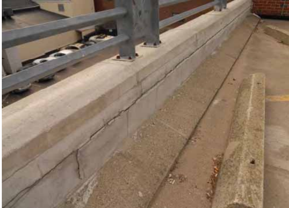
Photo 25 South Elevation. Interior view of CMU masonry wall at "A" line with damage and deterioration.
