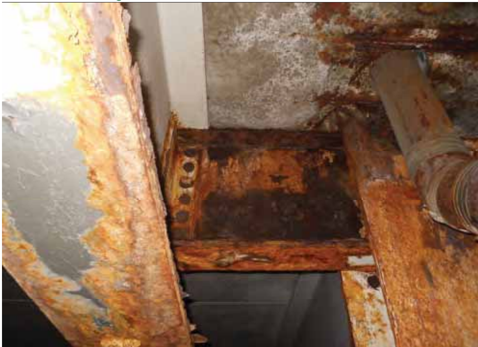
Photo 22 Sever corrosion formation (hot spots) on painted structural framing.
