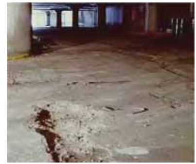
EXTENSIVE FLOOR SLAB SPALLING
