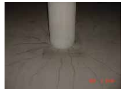
CRACKS RADIATING FROM COLUMN
