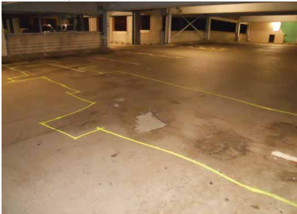
Photo 4 Level 3 – Deterioration in topping concrete. Note patching and spalls.
