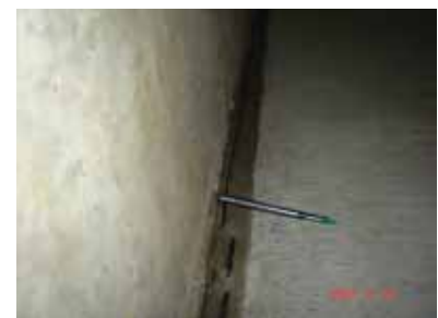
FAILED JOINT SEALANT
