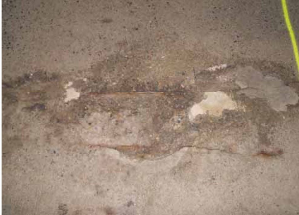
Photo 5 Typical concrete spalling with exposed corroded reinforcing steel near the surface.
