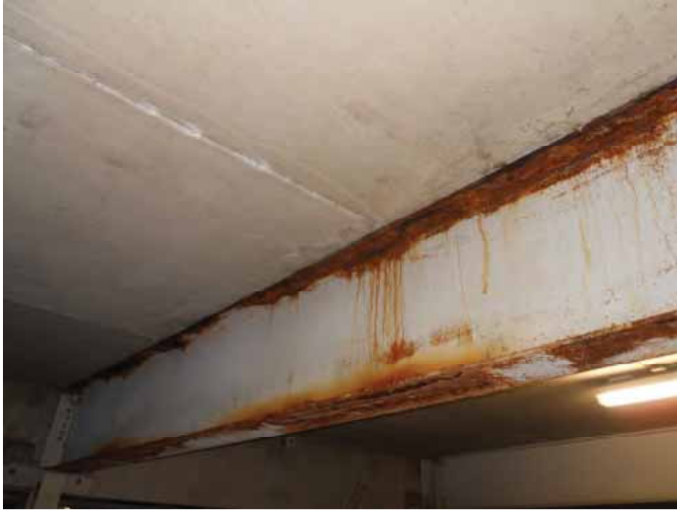
Photo 21 Typical corrosion formation on painted structural framing.
