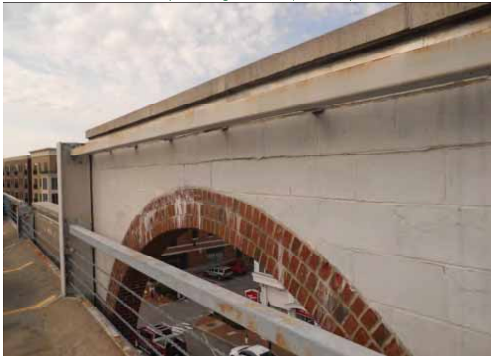
Photo 28 North elevation. Masonry brick and CMU wall showing deterioration (cracking, bond separation).
