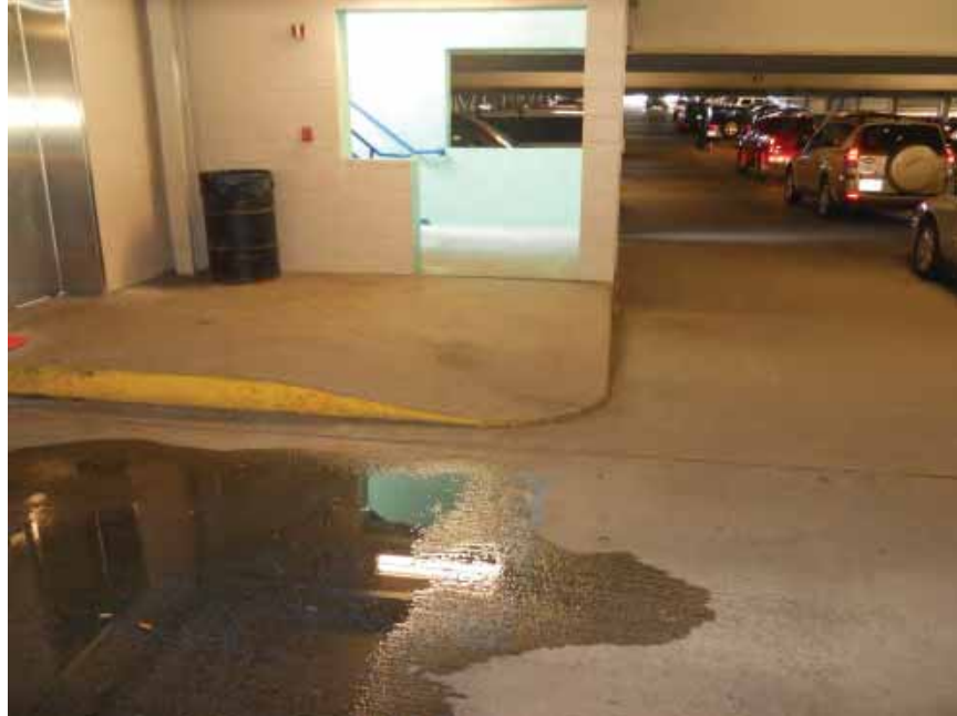
Photo 13 Level 2 – Landing area at stairtower/elevator. Note non-standard walkway drop and ponding near this area.
