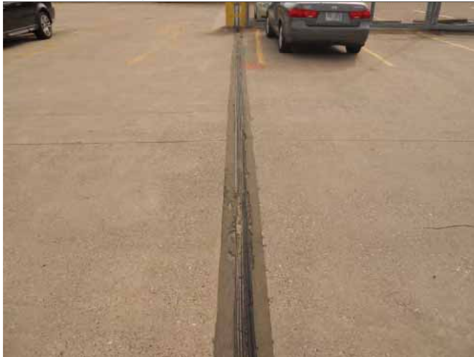
Photo 16 Expansion joint seal deterioration and damage.
