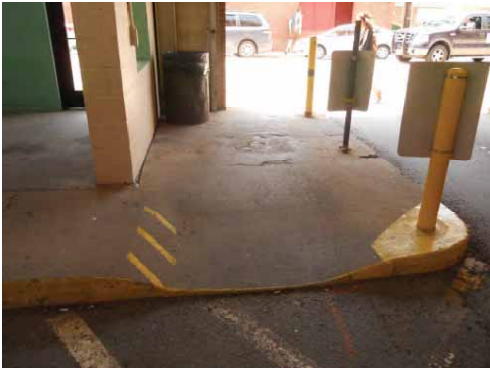
Photo 12 Level 2 – Deterioration on concrete walkway.
