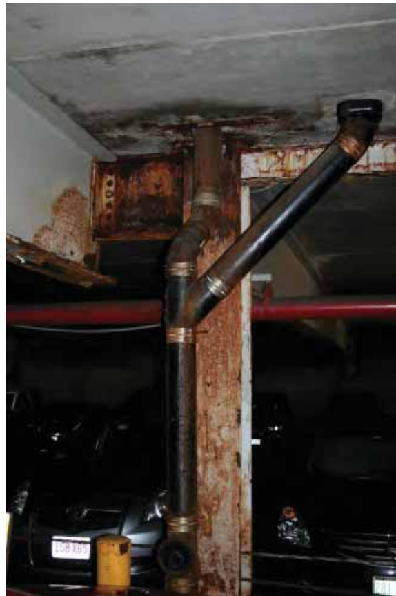
Photo 14 View of corrosion appearing on filigree planks, steel framing, and drain lines.
