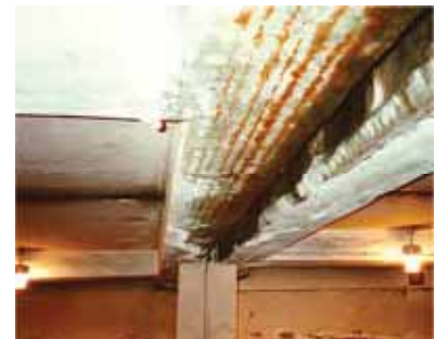
CORROSION OF REINFORCING STEEL IN/THROUGH CONCRETE BEAM
