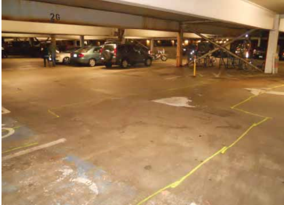
Photo 7 Level 2 – Large area of delaminated/debonded concrete topping.
