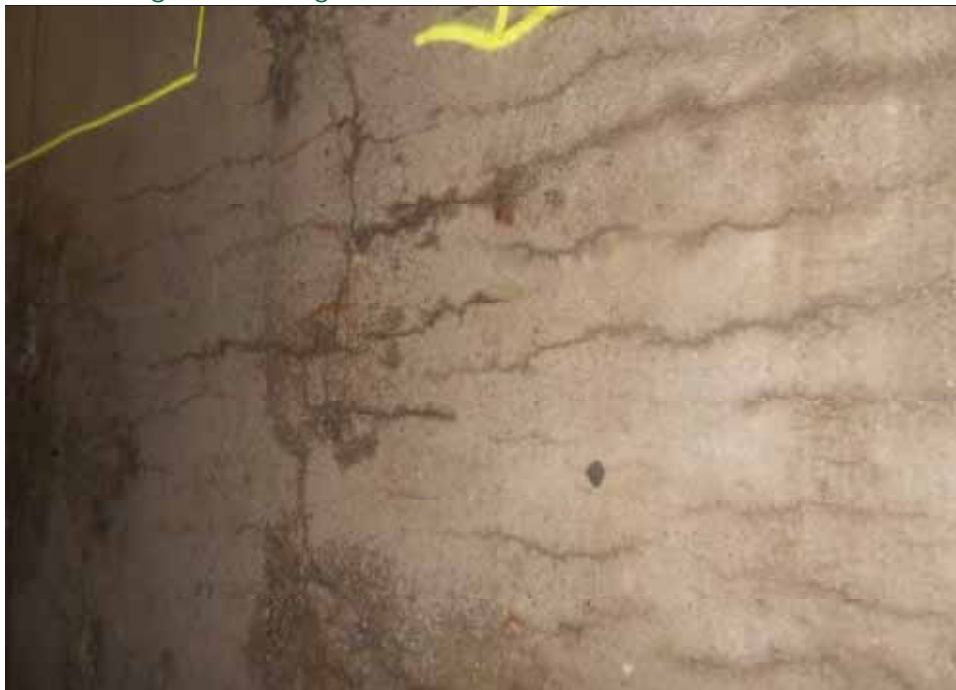
Photo 8 Typical flexural pattern cracking in topping concrete above girder framing.
