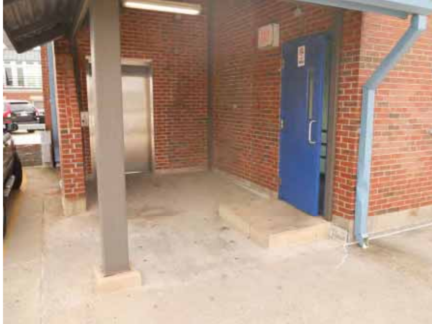
Photo 35 View of stairway access on Level 4. Note short landing slab at doorway.
