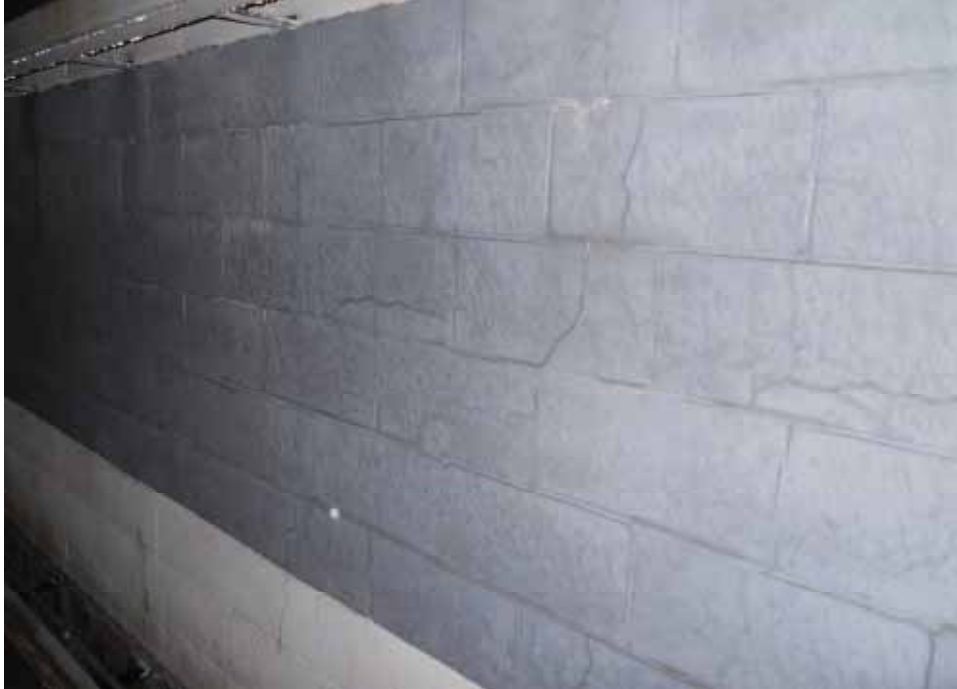
Photo 29 North Elevation. Interior view of cracking in CMU masonry façade.
