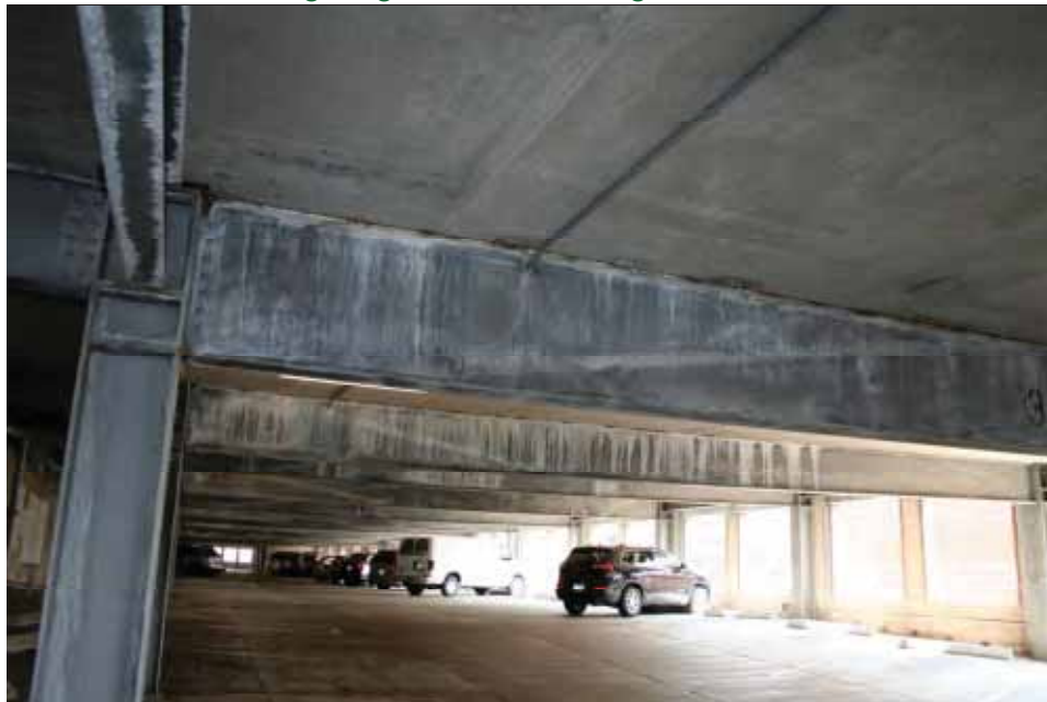
Photo 18 View of garage expansion area with efflorescence staining and rusting on galvanized framing.
