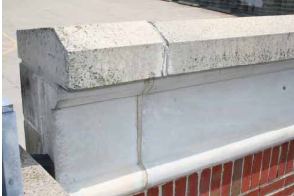
Photo 27 West Elevation. Stone cornice with mortar bond separation (typical)
