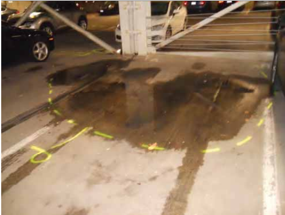
Photo 11 Level 2 – Large area where floor ponding exists.
