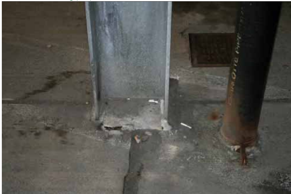
Photo 20 Level 4 – Floor expansion area. View of floor penetrations lacking proper seal.
