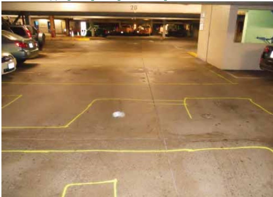
Photo 6 Level 3 – Large area of delaminated/debonded concrete topping along steel girder framing.
