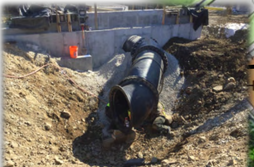
The existing force main from the Mechanic Street Pumping Station will connect to the new piping shown here at the Headworks Building. This will require temporarily maintaining wastewater flow during this work. This work is anticipated in the 2nd quarter.
