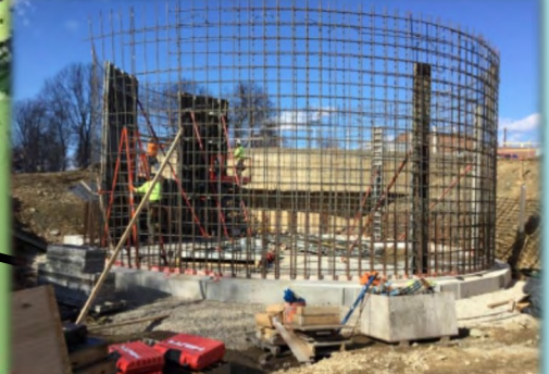
Rebar installed for the walls of Sludge Thicker No. 2 ("GT2"). Installation of forms and placement of walls are the next steps. This structure will temporarily house pumps while the new buildings are constructed.
