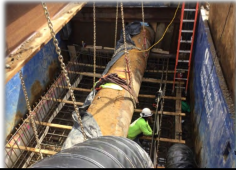
Excavation and concrete work for a valve vault for the magnetic flow meter in a 36" diameter pipe.
