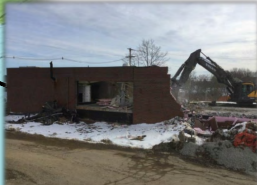
The original Filter Building constructed in 1985 was demolished and the new BAF facility will be located in this area. The hole for the new BAF facility will extend approximately 27-feet deep.
