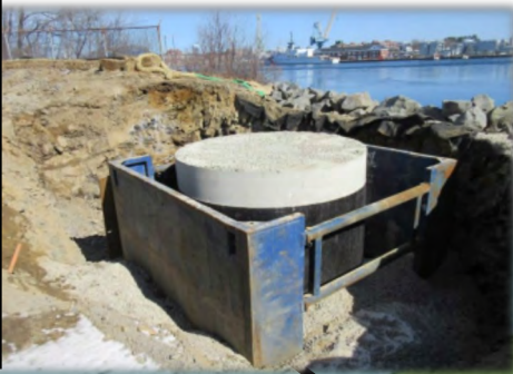
Installation of a sanitary pump station to serve solids handling recycle streams.
