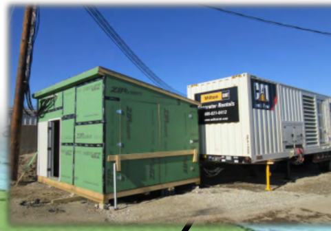
The Contractor installed temporary power to allow for the demolition of the original Filter Building. The temporary electrical service required a standby generator and rewiring electrical facilities to all buildings.
