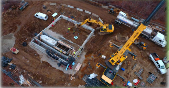
Construction of the foundation and channels for the new Headworks Building. The new Headworks will house screens that will remove toiletries and other debris in the wastewater. These screens will protect the downstream Biological Aerated Filter (BAF) process.
