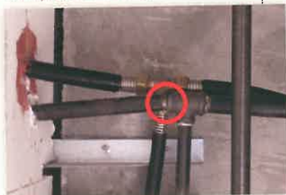
The black iron pipe, which was installed next to CounterStrike, fractured in the same test. It took 96 man hours to install the black iron pipe versus just 32 man hours to install CounterStrike.
