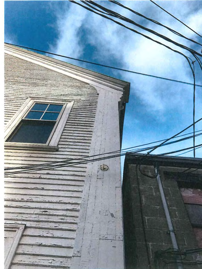
"GAP" AT REAR OF WOOD STRUCTURE SEEN FROM PORTER ST.
