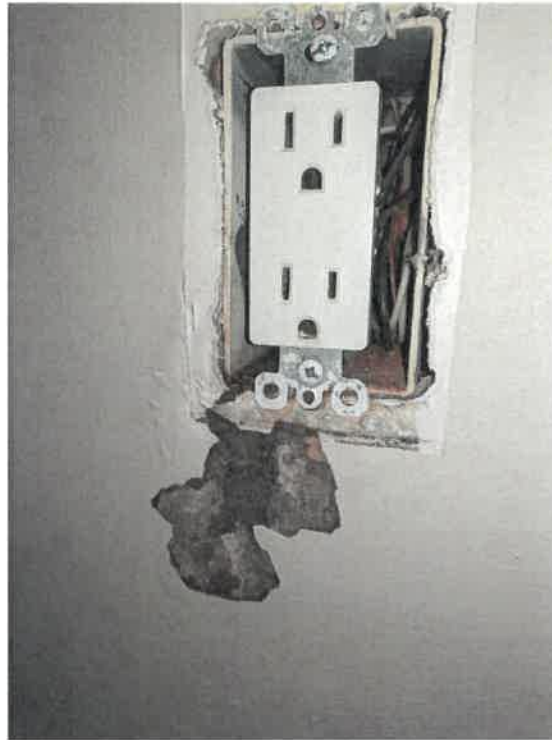
3/9/2018 | First signs of water and mold in March 2018
