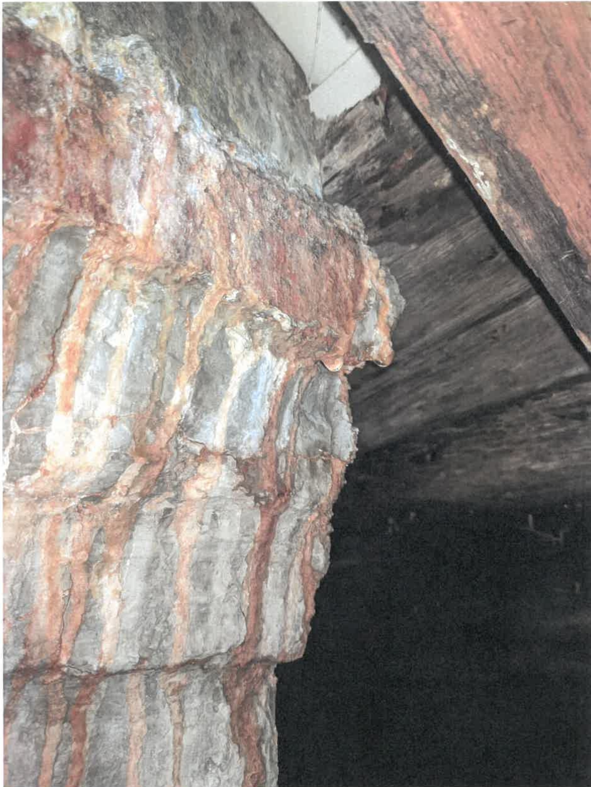
11/24/2019 | Interior view of chimney in attic, water droplets visible
