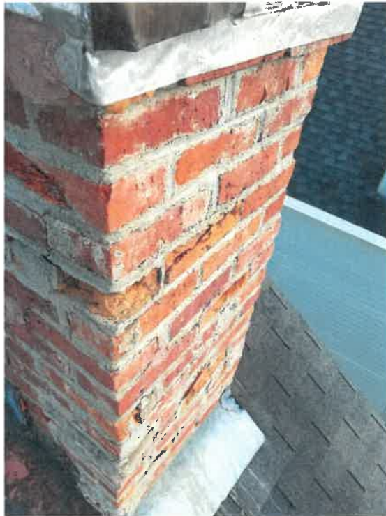
4/10/2018 | Brick has become brittle and porous
