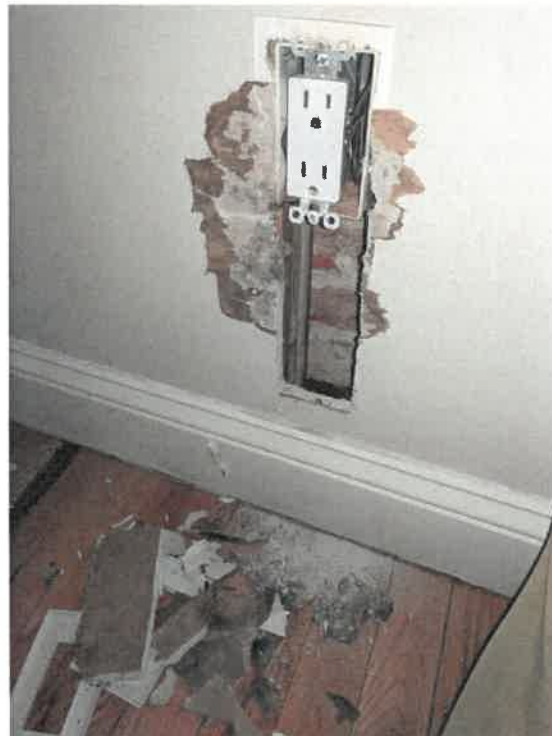
3/9/2018 | Mold and damaged drywall, the brick chimney can be seen through the drywall.
