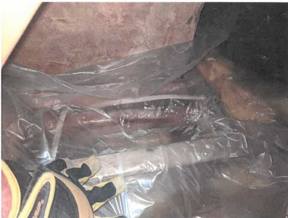
11/25/2019 | Water collected in ~2 hours after hearing water dripping down the walls
