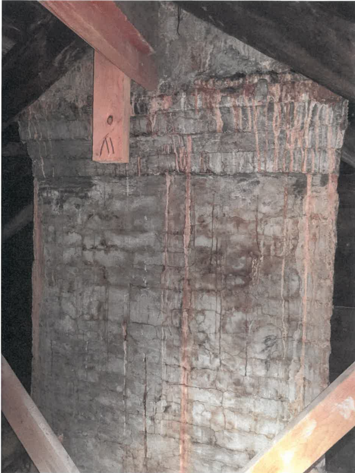
11/25/2019 | Interior view of chimney in attic, mineral deposits from water intrusion visible
