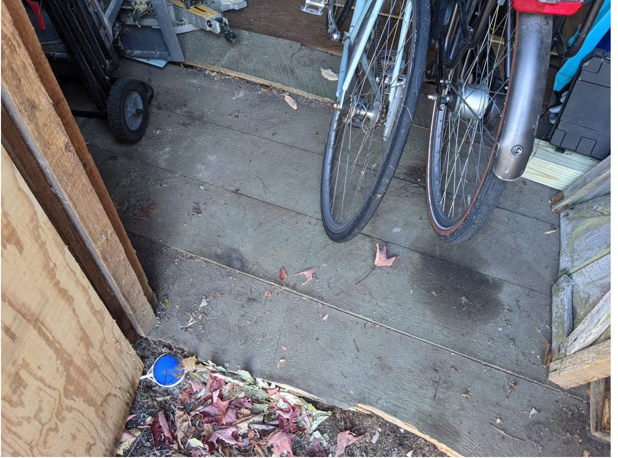
Inside shed, its rotting and needs replaced.
