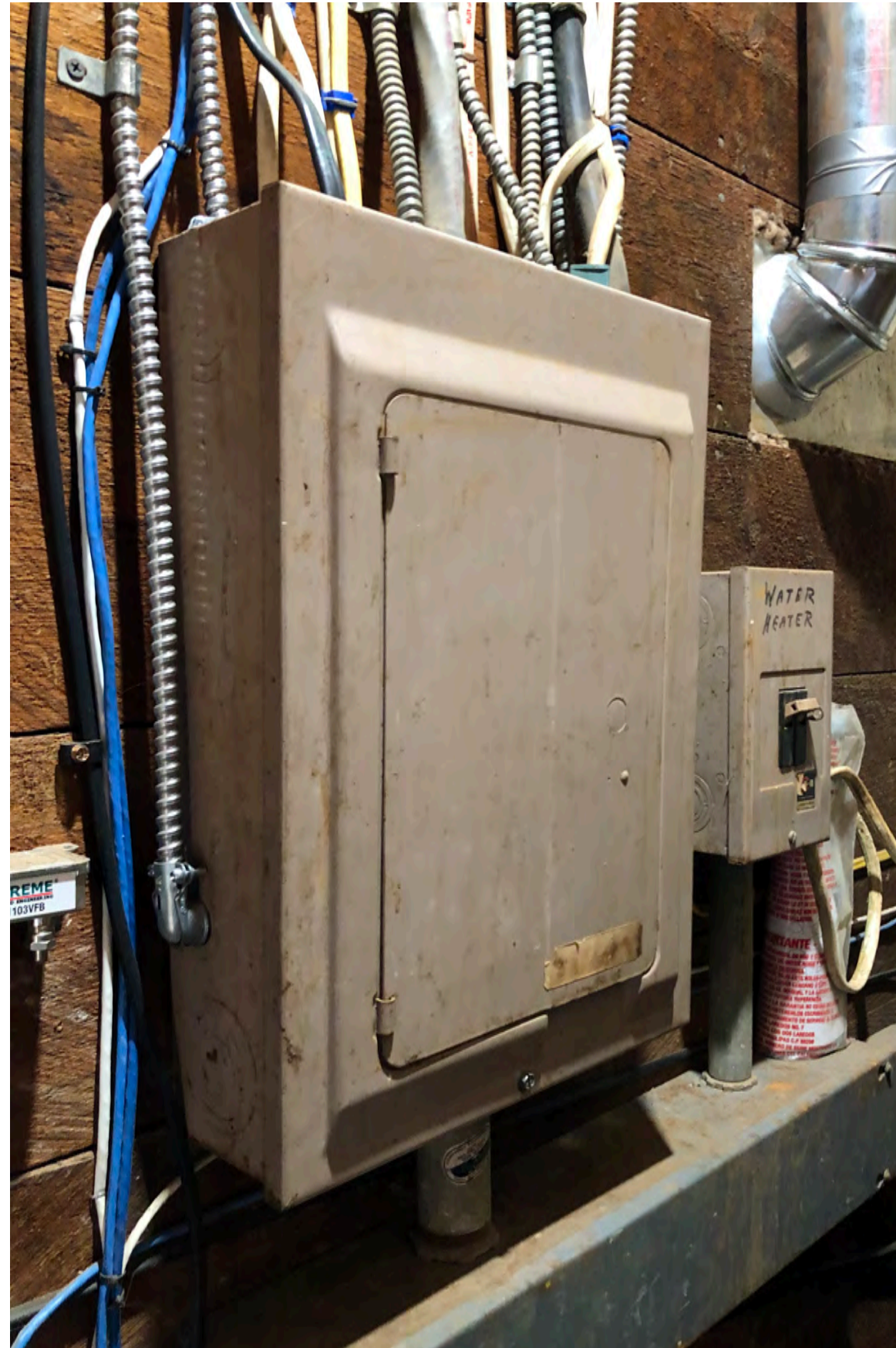
Shaw 1st Floor - Electric Panel
