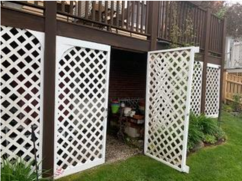
Condenser screening: (under deck)
