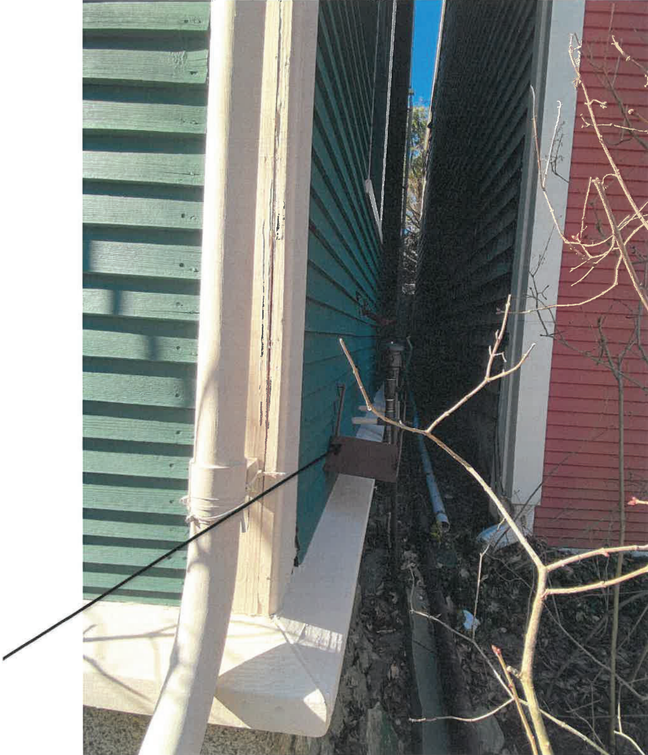
Close Frontal View (vent at location of hose reel, which would move forward to hide vent):
