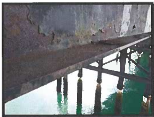
Typical Beam Corrosion
