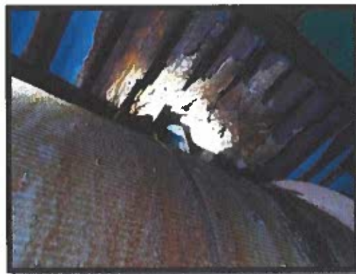
Deck Spall at Northern Air Release Valve
