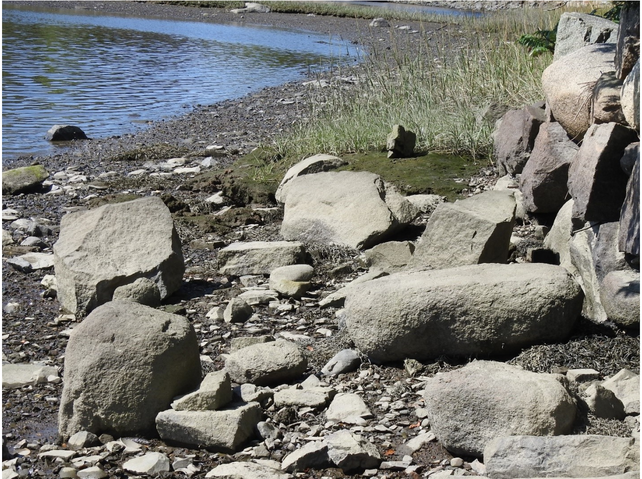
Union Cemetery Deterioation of Retaining Stone Wall
