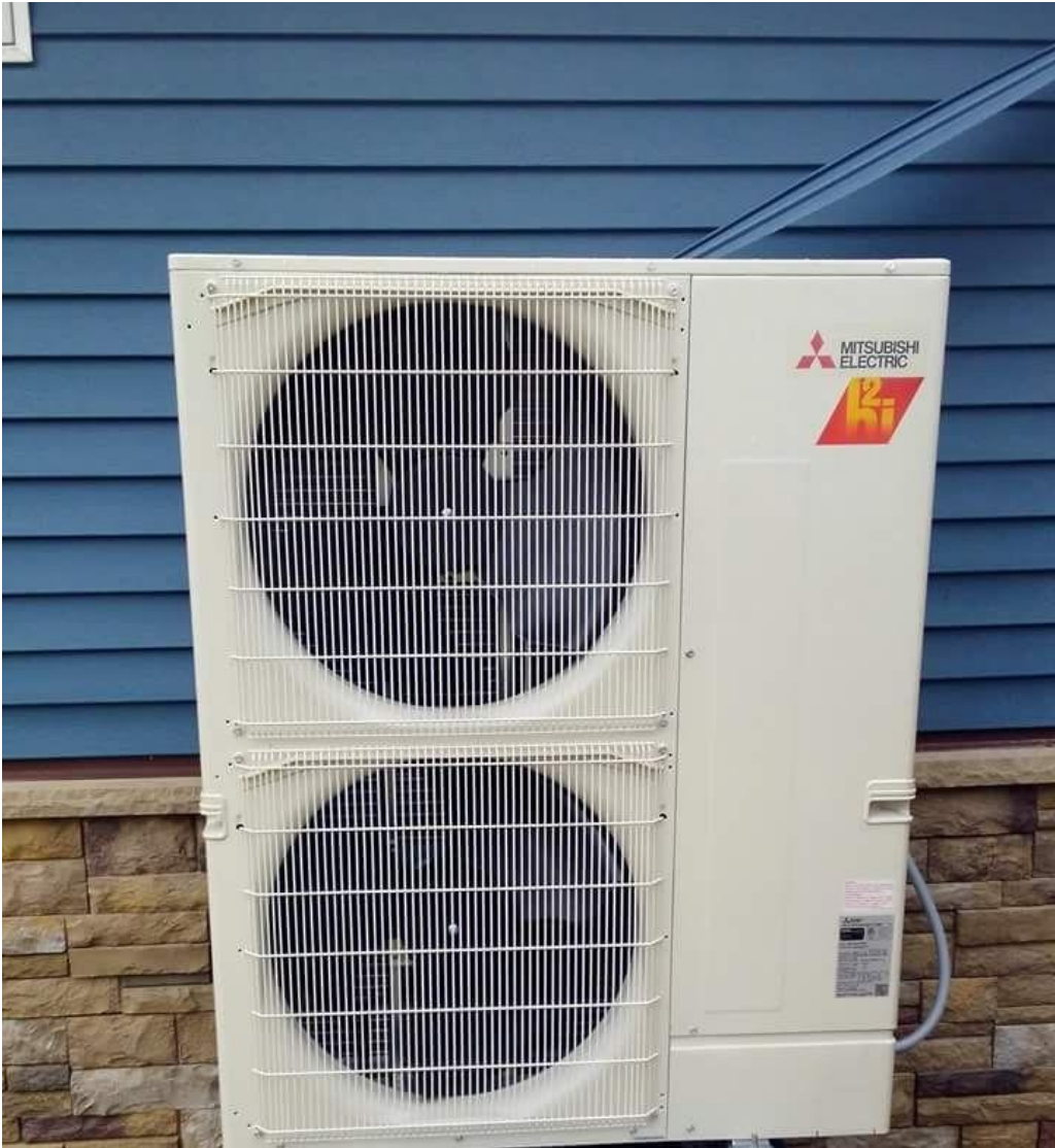
MITSUBISHI HEAT PUMP:
