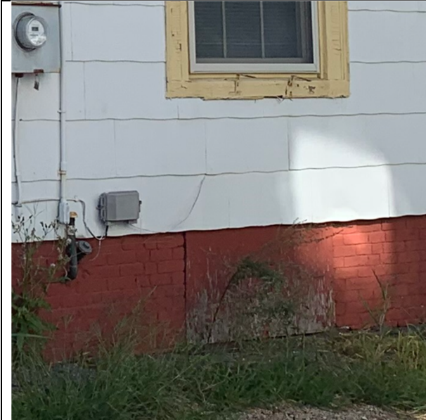
Original Basement window opening boarded up
