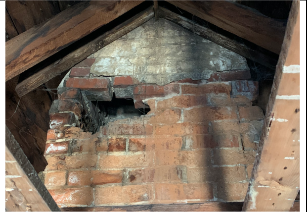
Hole in chimney, brick in poor condition
