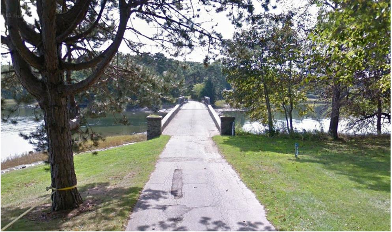
Photo 5. A final view of the bridge approach on Lady Isle to be replaced as well as a portion of upland.
