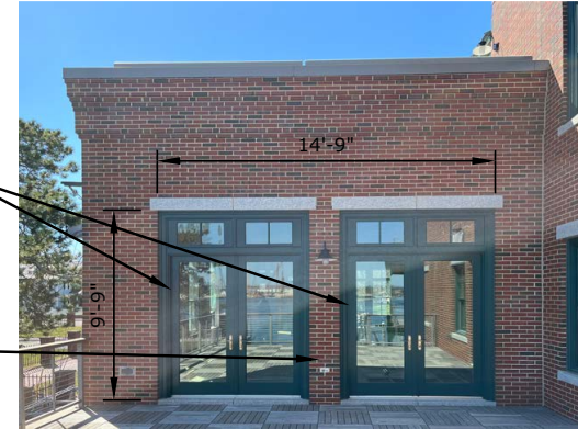
2 EXISTING FAILING TERRACE DOORS (PHOTO) Scale: NONE
