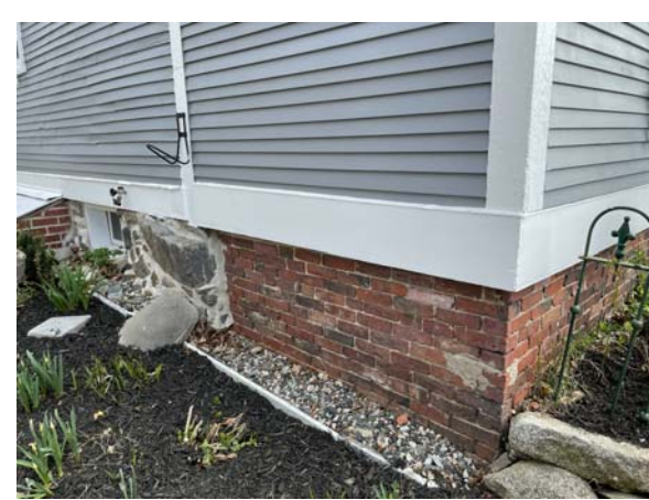
DESIGN INTENT: MATCH EXISTING BASE TRIM, WOOD CLAPBOARD, AND BRICK FOUNDATION AT PROPOSED ADDITIONS
