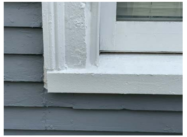
DESIGN INTENT: MATCH EXISTING WOOD WINDOW TRIM AND SILL PROFILES AT PROPOSED WINDOWS
