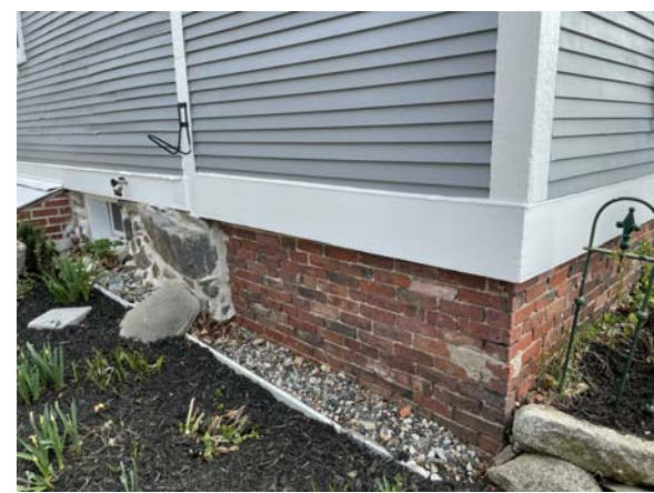
DESIGN INTENT: MATCH EXISTING BASE TRIM, WOOD CLAPBOARD, AND BRICK FOUNDATION AT PROPOSED ADDITIONS
