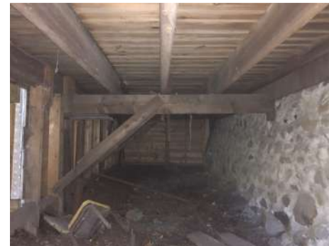
EXISTING UNDERSIDE OF PORCH WITH CENTRAL SUPPORT BEAM & RUSTING LALLY SUPPORTS
