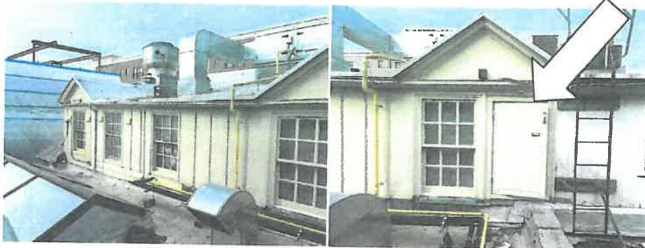
View of roof dormer. Arrow points to door to be replaced by new window to match adjacent original windows.
