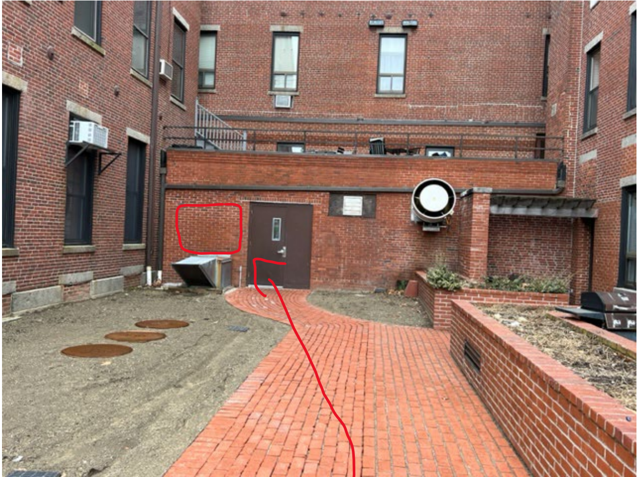
Existing Unit Location+ Location of new condenser.
