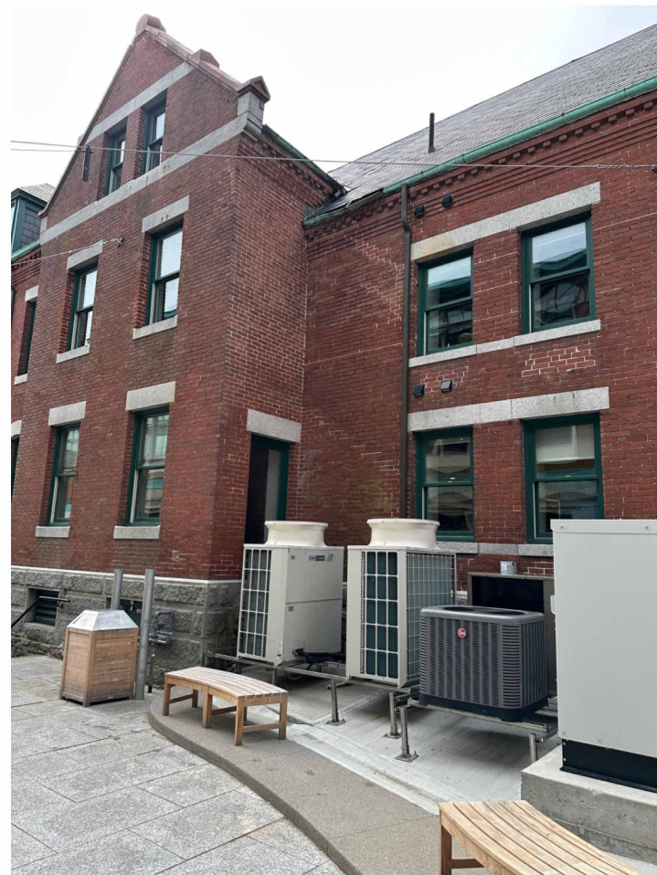
EXISTING COMPRESSOR TO BE COVERED
