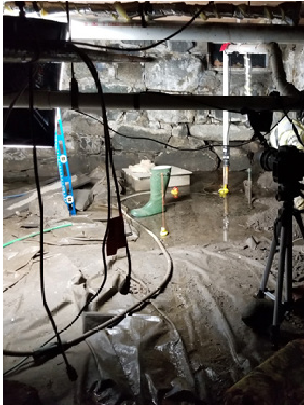
FLOODING AT PENHALLOW REAR
