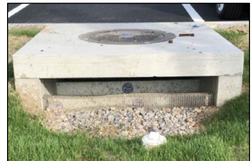
REAR VIEW OF OUTLET SCREEN
