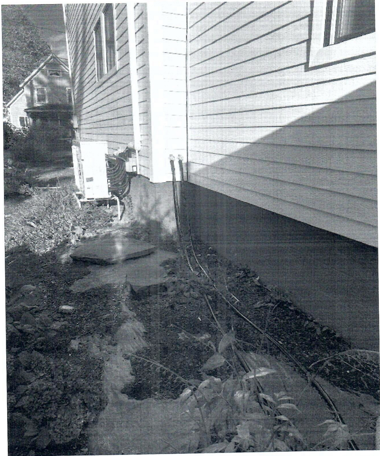
Site Photos—Exhibit B-4: Photo #2 Right side of House / Current Mini Split Condenser
