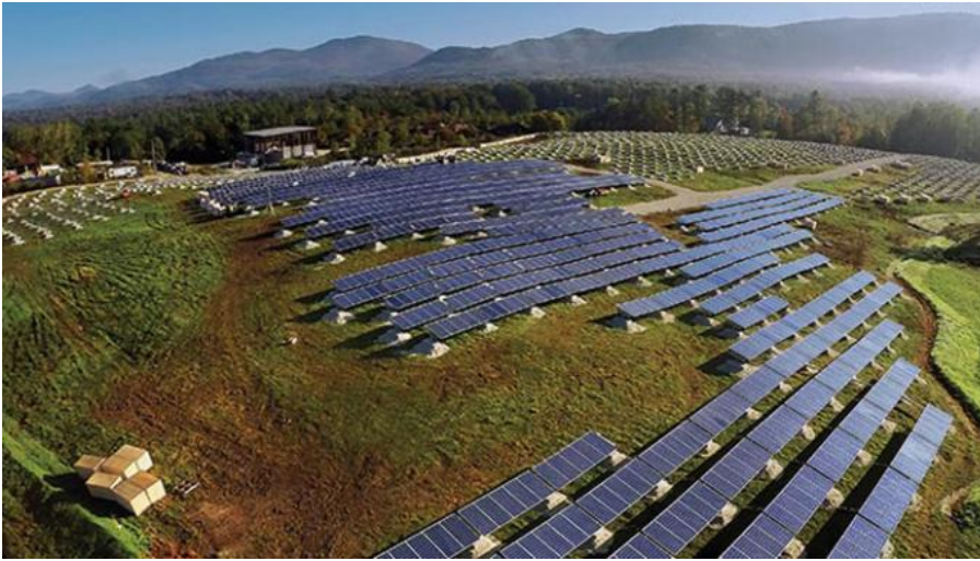
Green Mountain Power and the City of Rutland have installed the Stafford Hill plant (Left). This is a solar and battery system that can disconnect from the grid and supply critical power to an emergency shelter during long outages.
