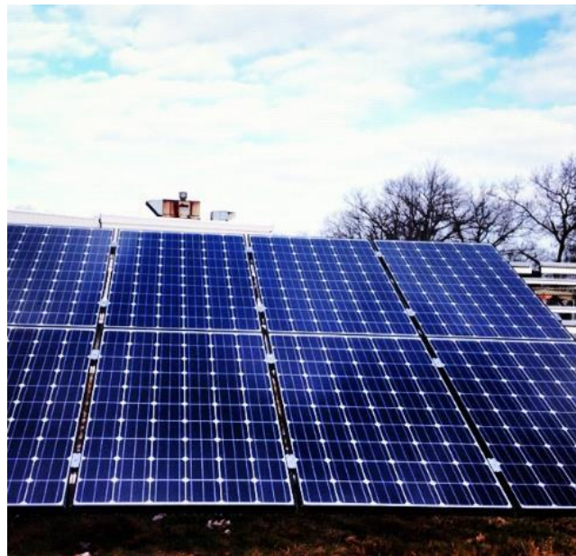
Completed installation showing gaps between panels
