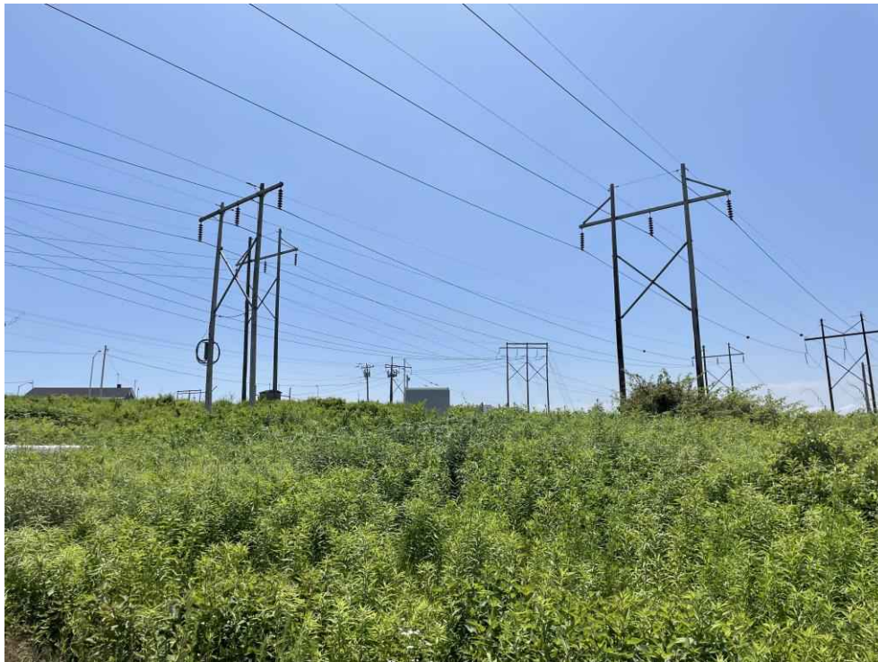
Photograph No. 22: Looking south near Wetland PW-2 (PEM1/PSS1E) on the T13 Line ROW off Gosling Road, Portsmouth, NH.
