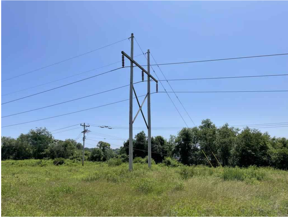
Photograph No. 29: Looking south at Structure 5 on the T13 Line ROW off Gosling Road, Portsmouth, NH.
