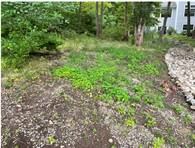
Figure 1. Downstream end of swale and discharge by improved stone wall end (top left); stone swale looking upstream, photo taken from area close to stone wall end (right); property directly north of swale subject to erosion, looking upstream, photo taken from area close to stone wall end (lower left).
