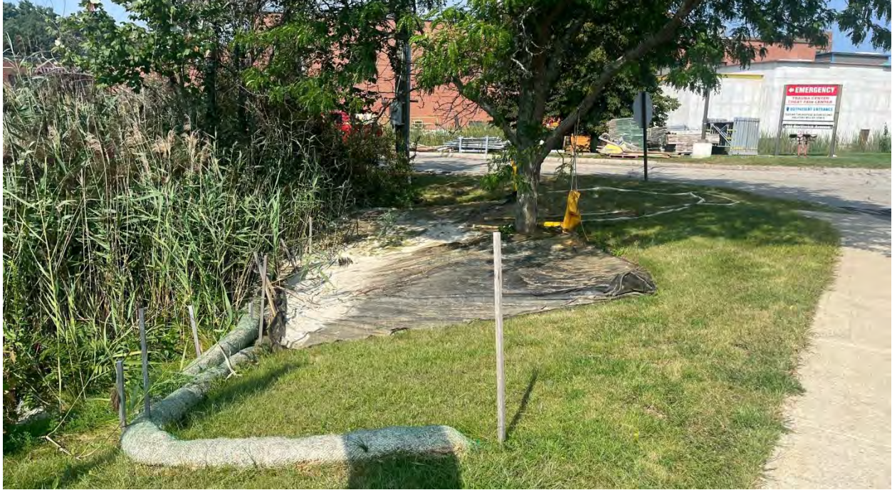
Photo #1: Looking at the dewatering system that doesn't appear to be in use anymore.
