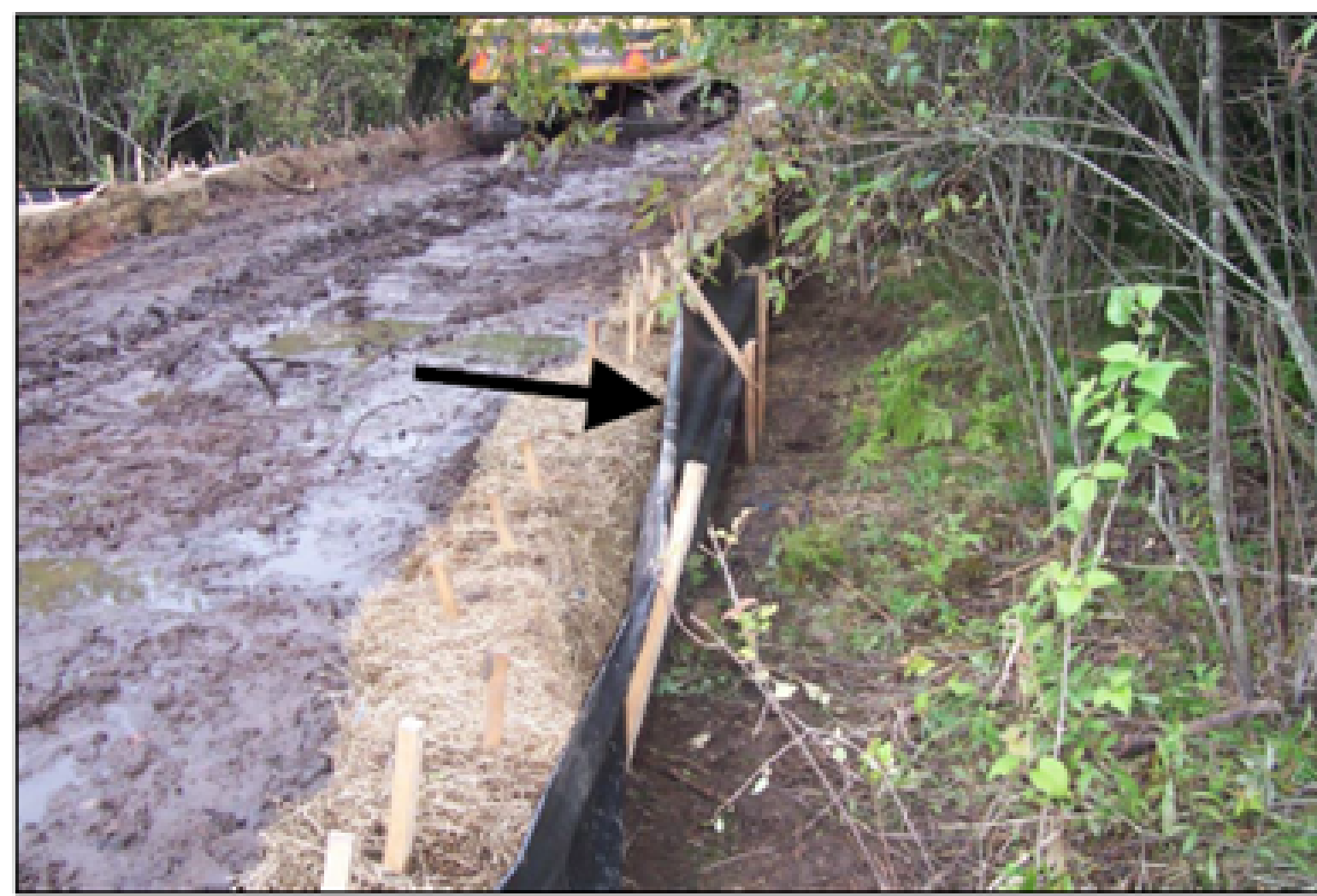
Properly installed hay bale barrier with silt fence (direction of flow indicated by arrow).
