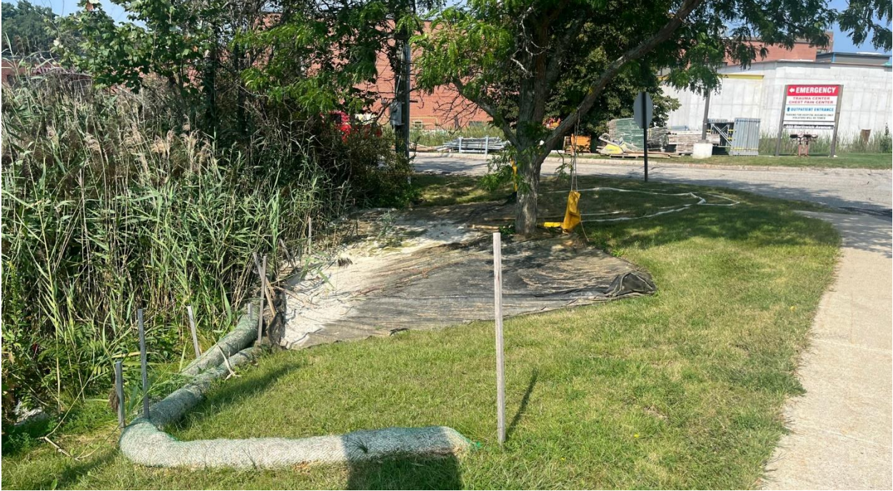
Photo #1: Looking at the dewatering system that doesn't appear to be in use anymore.
