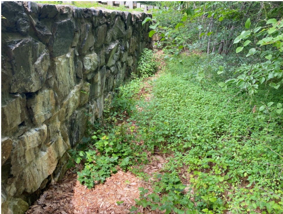
Photo 14. Overview of the undelineated area and the inflow on eastern side of Odiorne Point Road that flows to the northern culvert outflow into POGW2 shown in Photo 16, viewing north. (08-11-22)
