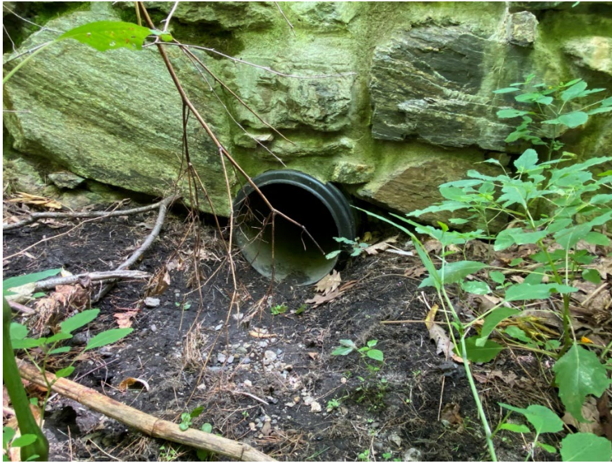
Southern culvert outflow serving as the delineated upstream end of POGS1 in wetland POGW2. (08-11-22)
