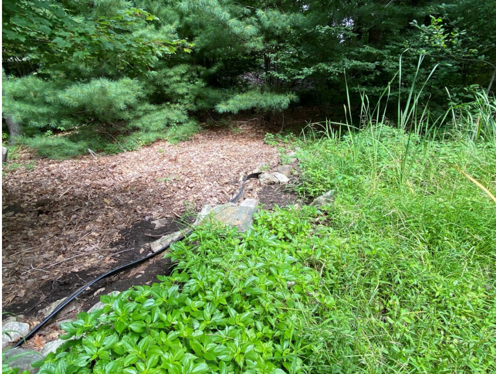
Photo 25. Plastic landscaping barrier that funnels flow from POGS1 into the upper portion of the stone swale, viewing north. (08-11-22)
