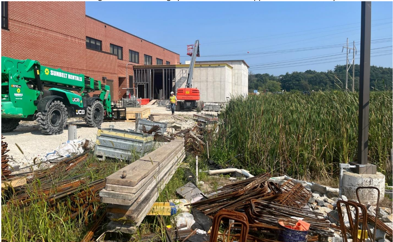
Photo #2: Looking at the continued construction at the location of the mobile unit.
