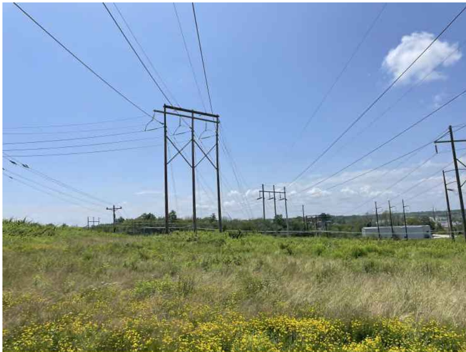
Photograph No. 22: Looking southwest at Structure 2 on the T13 Line ROW off Gosling Road, Portsmouth, NH.
