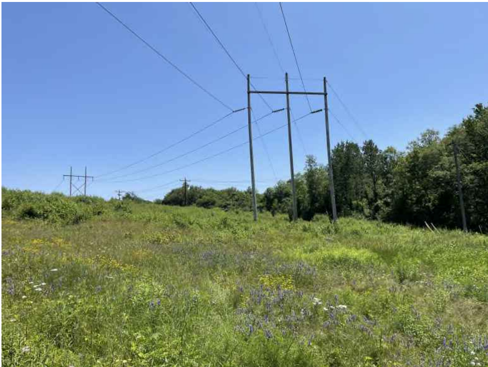
Photograph No. 26: Looking southeast at Structure 4 on the T13 Line ROW off Gosling Road, Portsmouth, NH.
