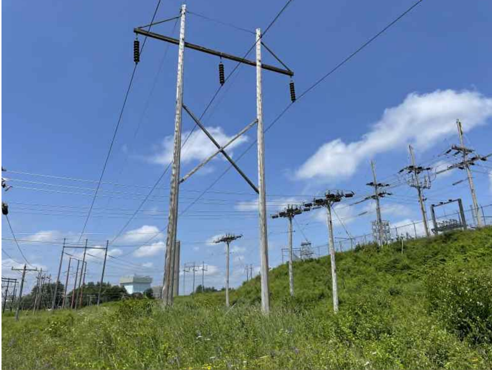
Photograph No. 25: Looking west at Structure 3.5 and Wetland PW-6 (PEM1/PSS1E) on the T13 Line ROW off Gosling Road, Portsmouth, NH.
