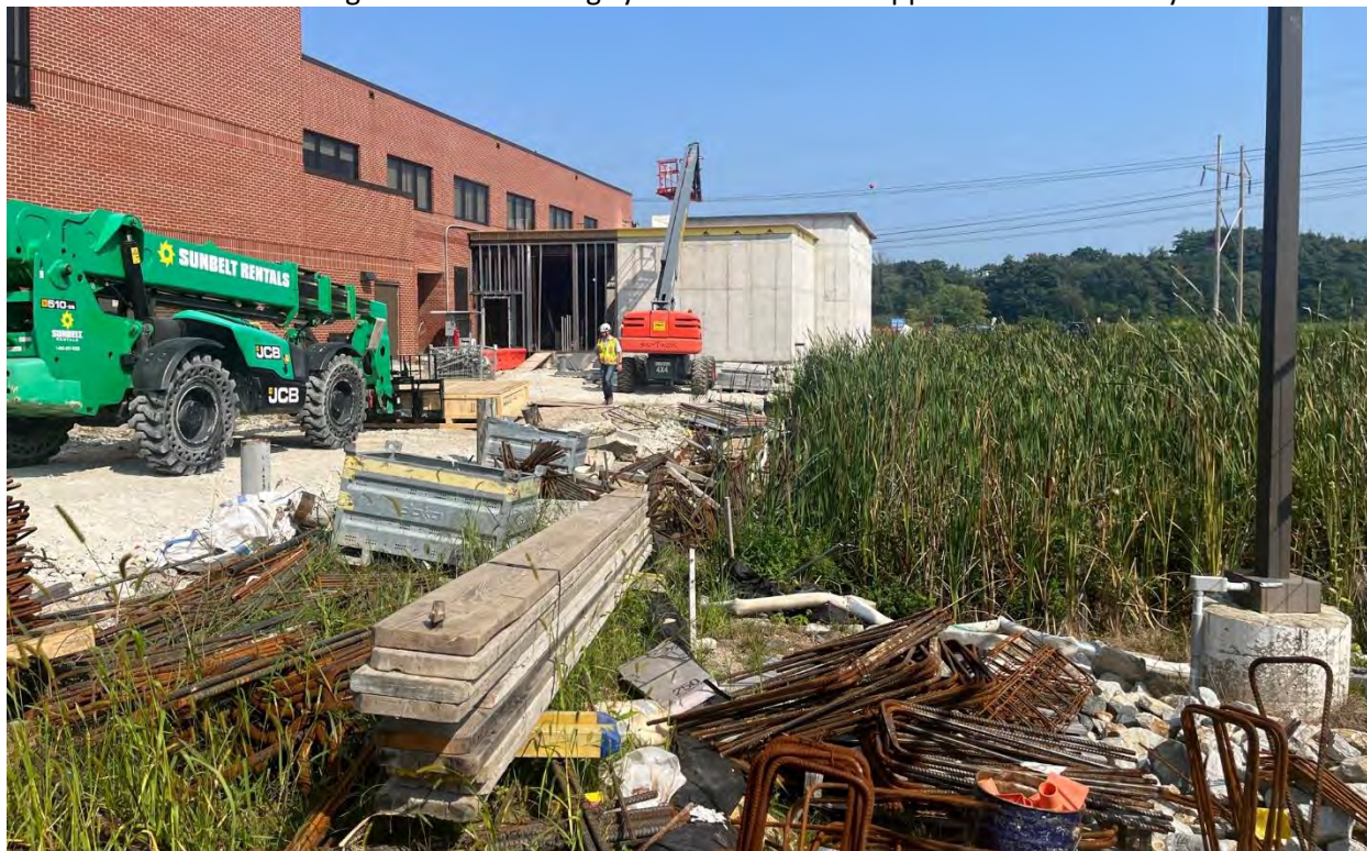
Photo #2: Looking at the continued construction at the location of the mobile unit.
