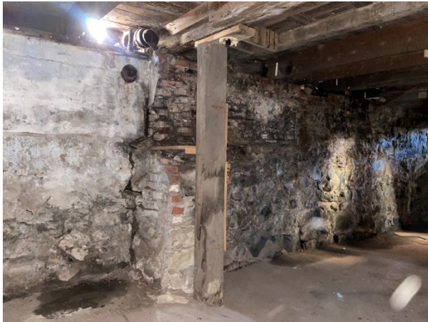
15-Timber post supporting decayed joist
