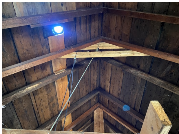
22-Cables connected to roof framing
