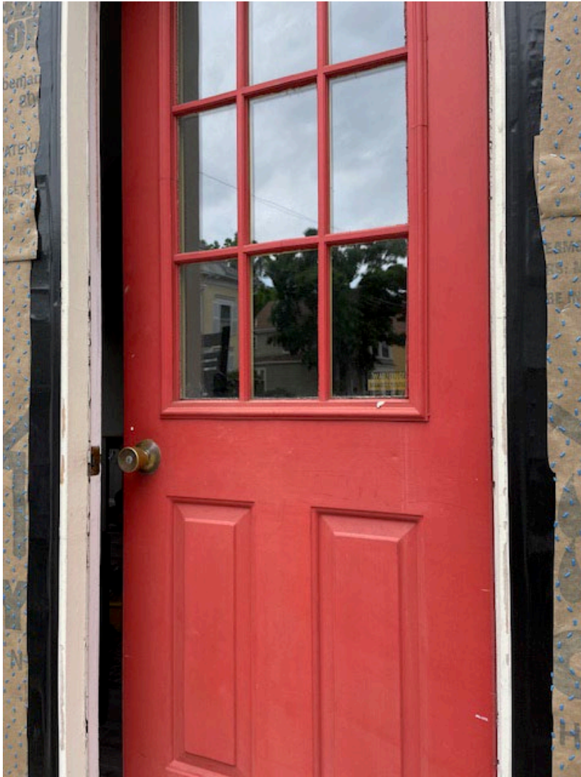
Existing front door to be replaced
