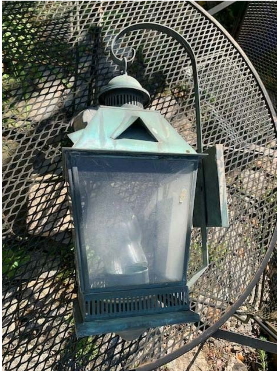
LT-6: WALL SCONCES AT REAR ENTRY DOOR AND DOOR TO ROOF DECK
