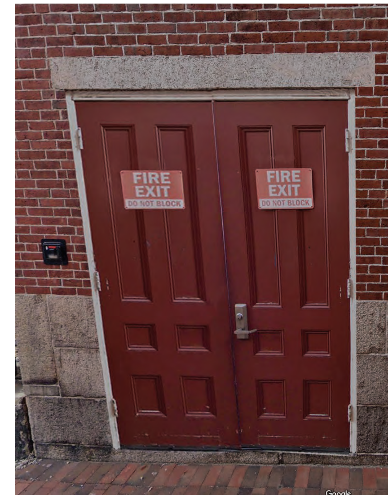
2A: PROPOSED REAR EGRESS DOUBLE DOOR ON PEDESTRIAN ALLEY Door widened to meet current egress code requirements
