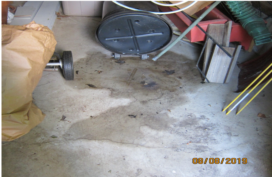
Illustration 1: Water in Basement Under New Addition
