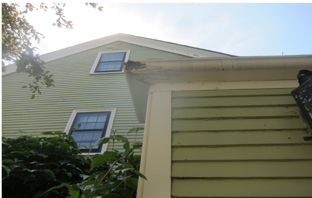
Rotted Gutter On Addition
