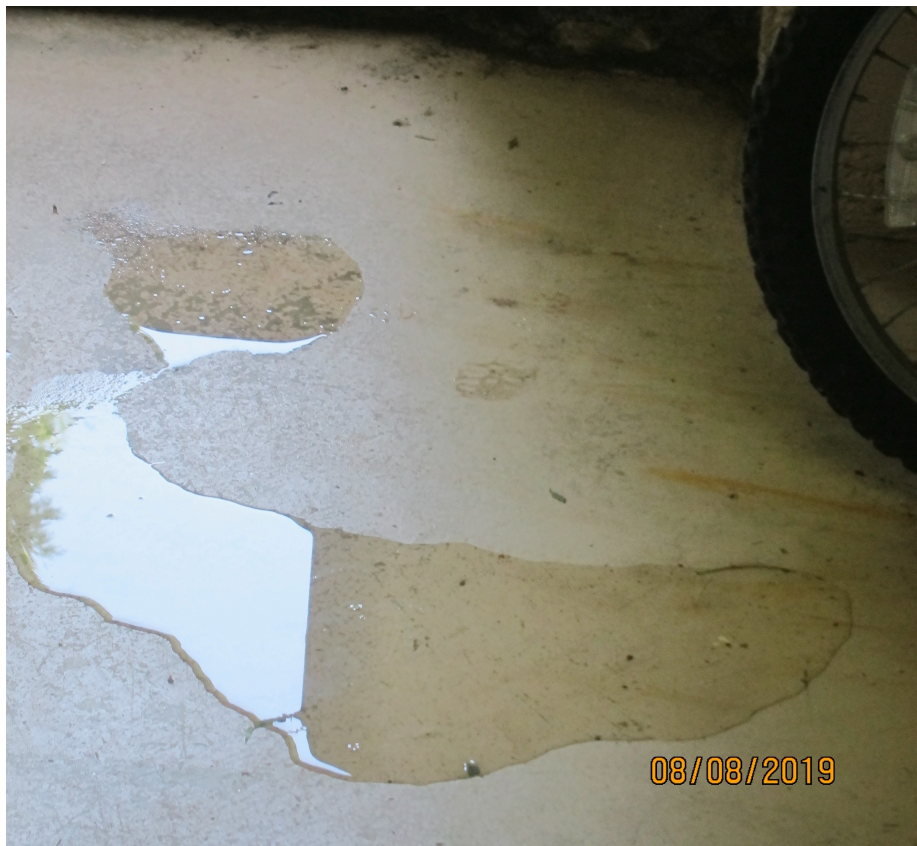
Illustration 2: Water in Basement Under the Main House
