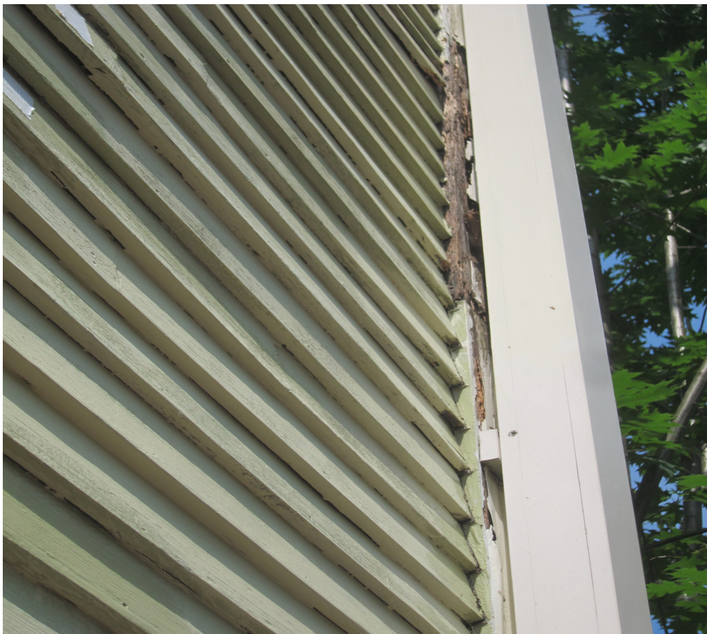
Rotted Cornerboard under front housedownspout. Low downspout capacity causes water to flow behind the downspout, rotting the board and siding underneath
