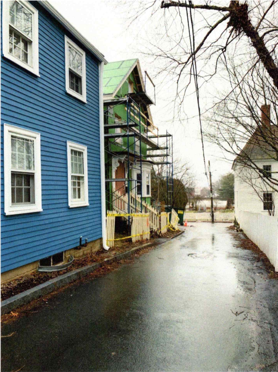
View of Solar Roof from Richmond Street
