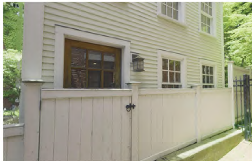
EXISTING ALLEYWAY FENCE OBSTRUCTING WINDOWS & DOORS
