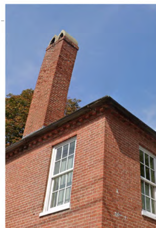
EXISTING UNSAFE LEANING CHIMNEY TO BE REMOVED & REBUILT. MATCH EXISTING HISTORICAL PHOTOS OF CHIMNEY & BISHOP'S CAP
