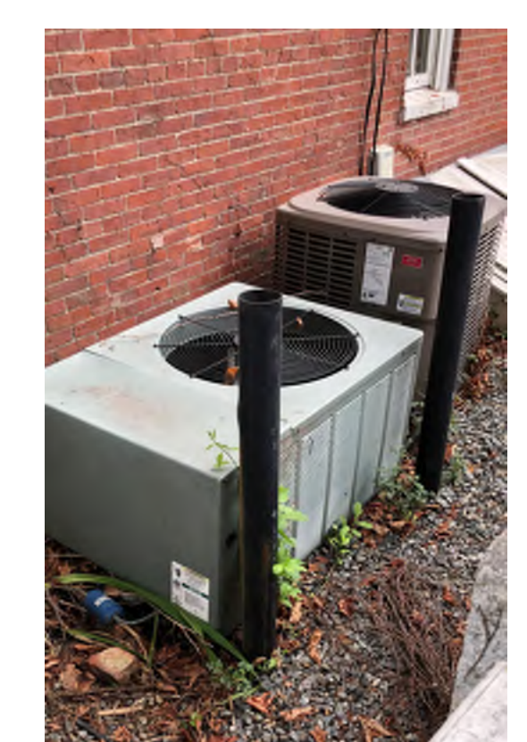
EXISTING HVAC UNITS
