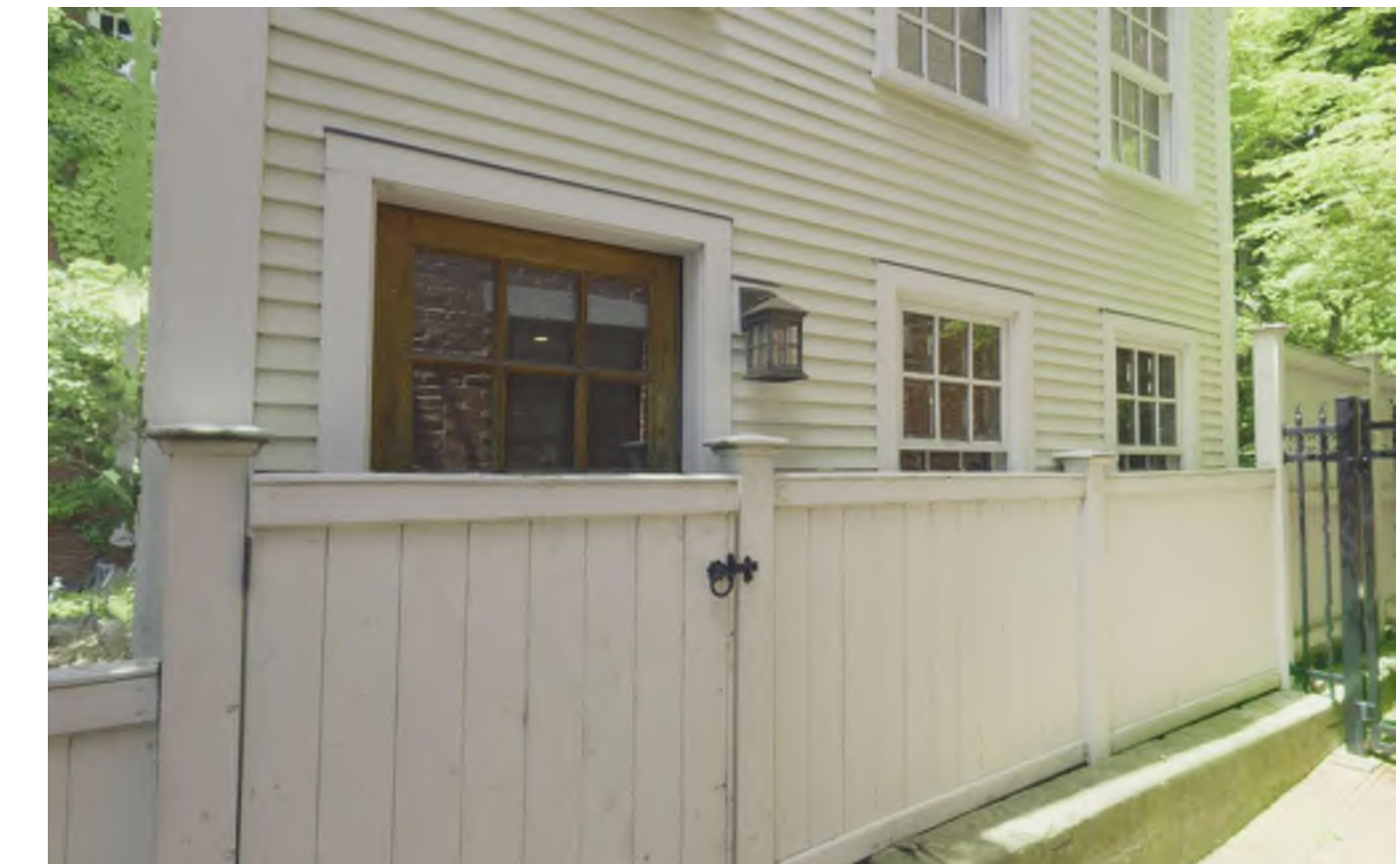
EXISTING ALLEYWAY FENCING OBSTRUCTING DOORS & WINDOWS - FIRST FLOOR ALLEYWAY DOORS & WINDOWS TO BE REMOVED & INFILLED
