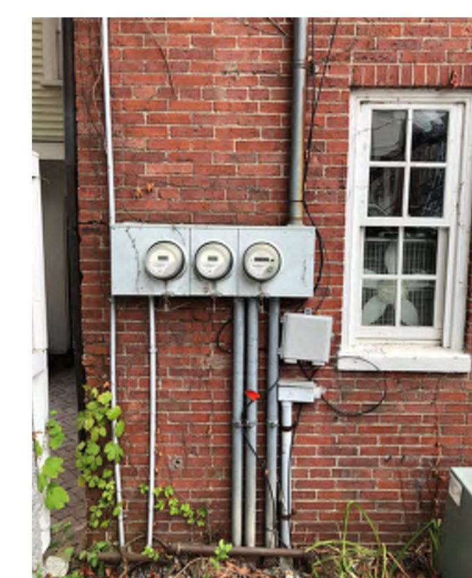
EXISTING ELECTRICAL METER
