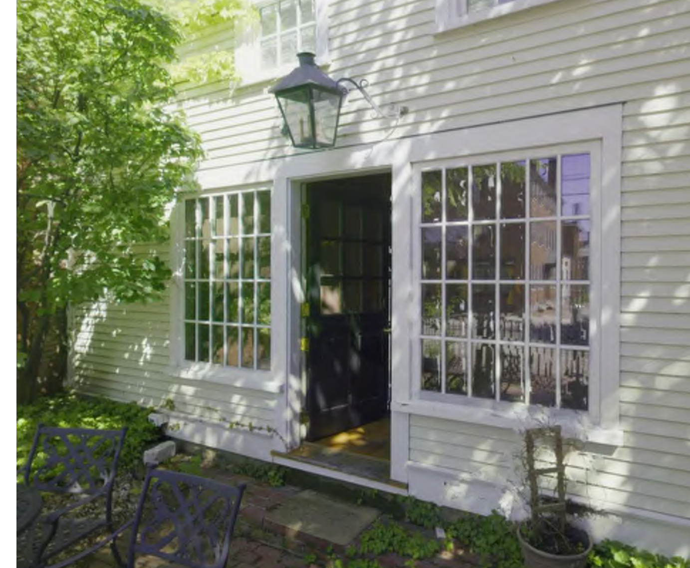
EXISTING DOOR 103 & WINDOW F ASSEMBLY CURRENT DOOR AND FRAME ALLOWS LIGHT, AIR AND WATER TO INFILTRATE
