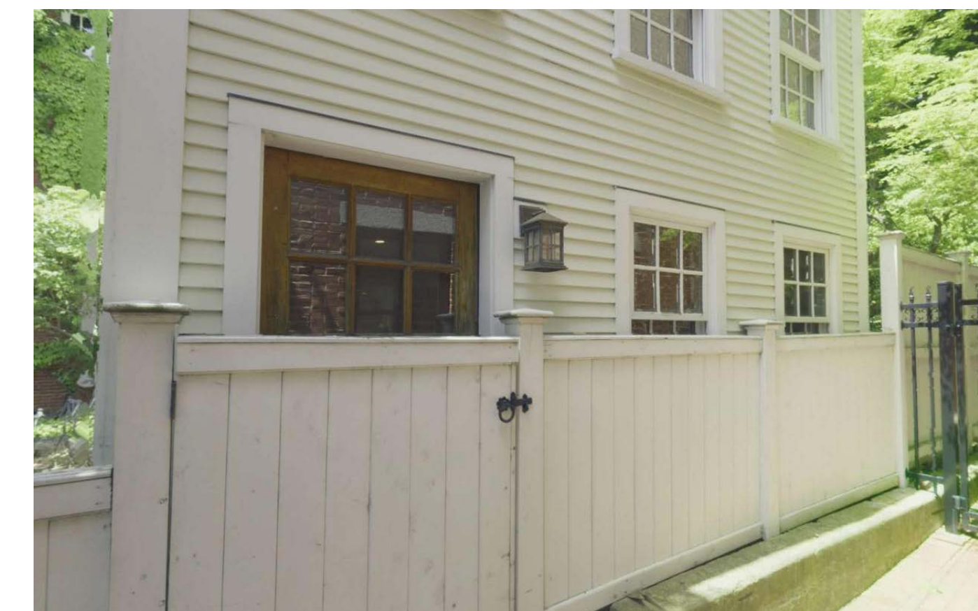
EXISTING ALLEYWAY FENCING OBSTRUCTING DOORS & WINDOWS - FIRST FLOOR ALLEYWAY DOORS & WINDOWS TO BE REMOVED & INFILLED
