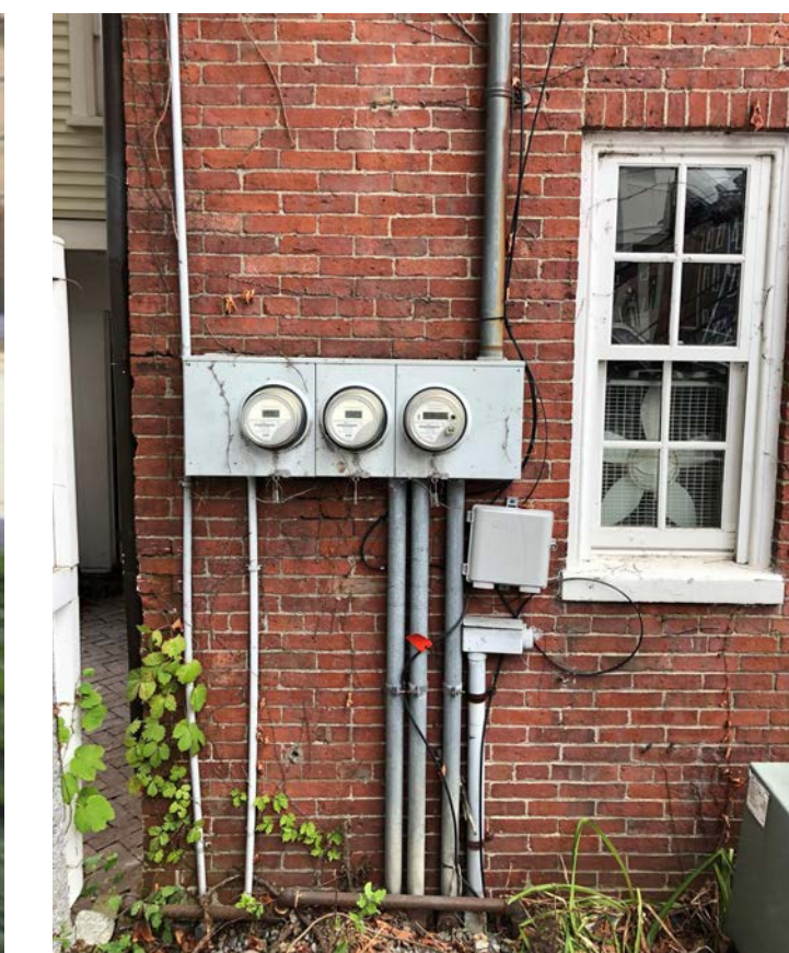
EXISTING ELECTRICAL METER
