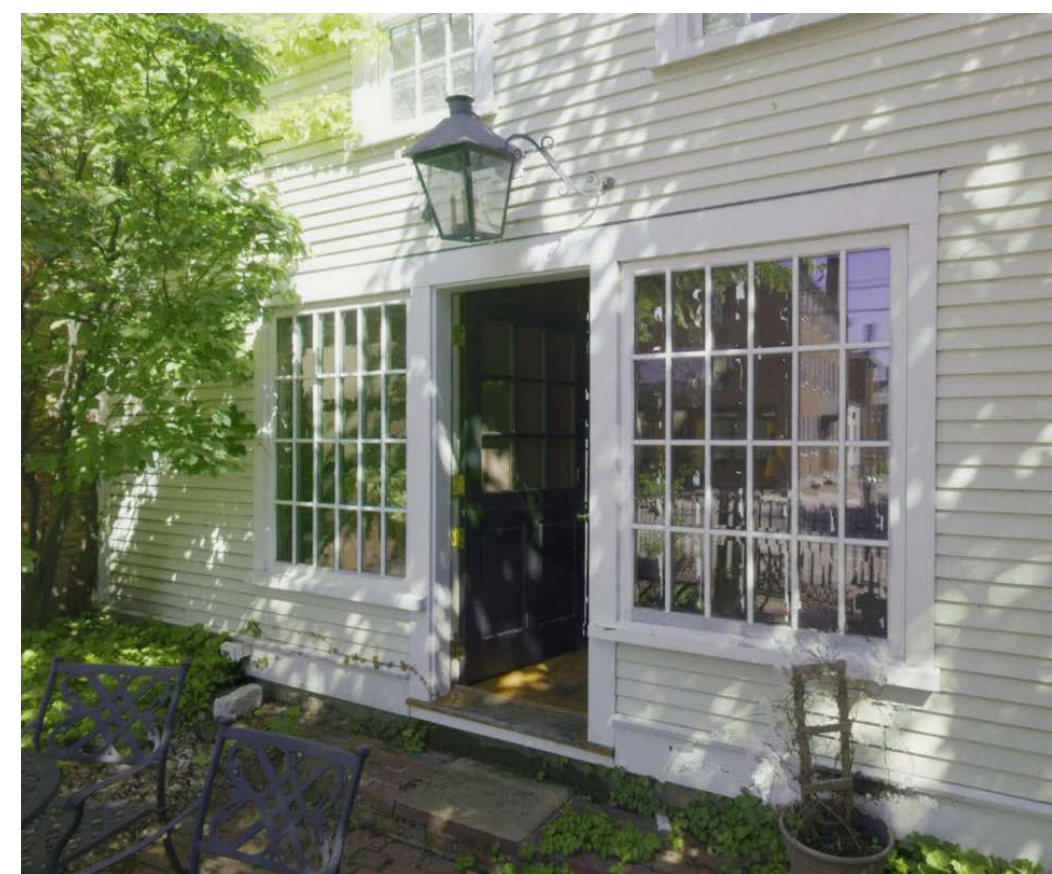
EXISTING CARRIAGE HOUSE ENTRY (STATE STREET FACADE) - BRICK STEP TO BE REPLACED W/ GRANITE
