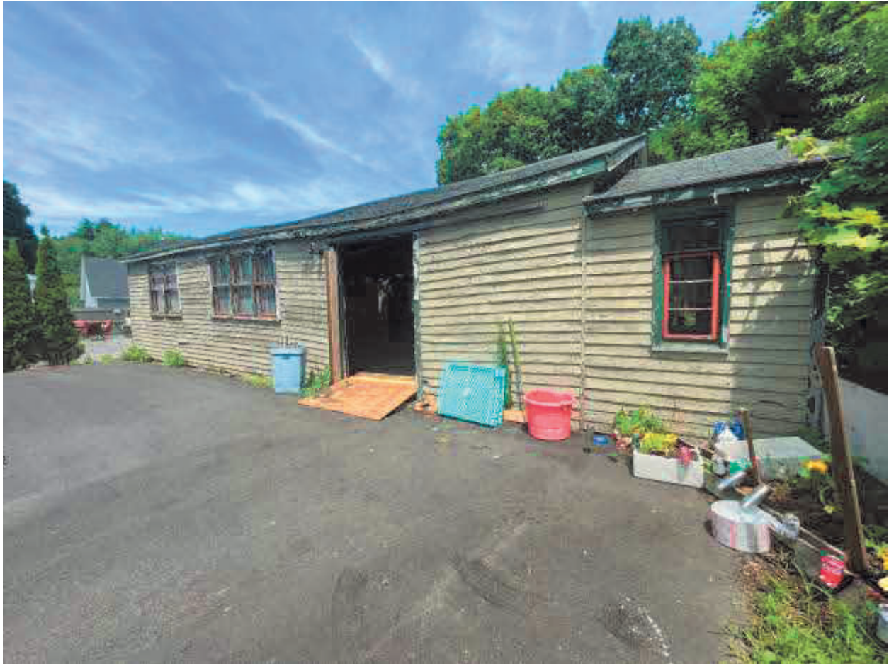
Accessory Building (Front View)
