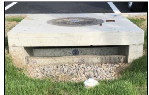
REAR VIEW OF OUTLET SCREEN
