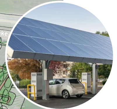
On-site solar PV ready
