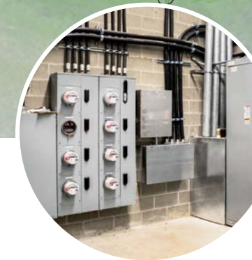
All electric building systems
