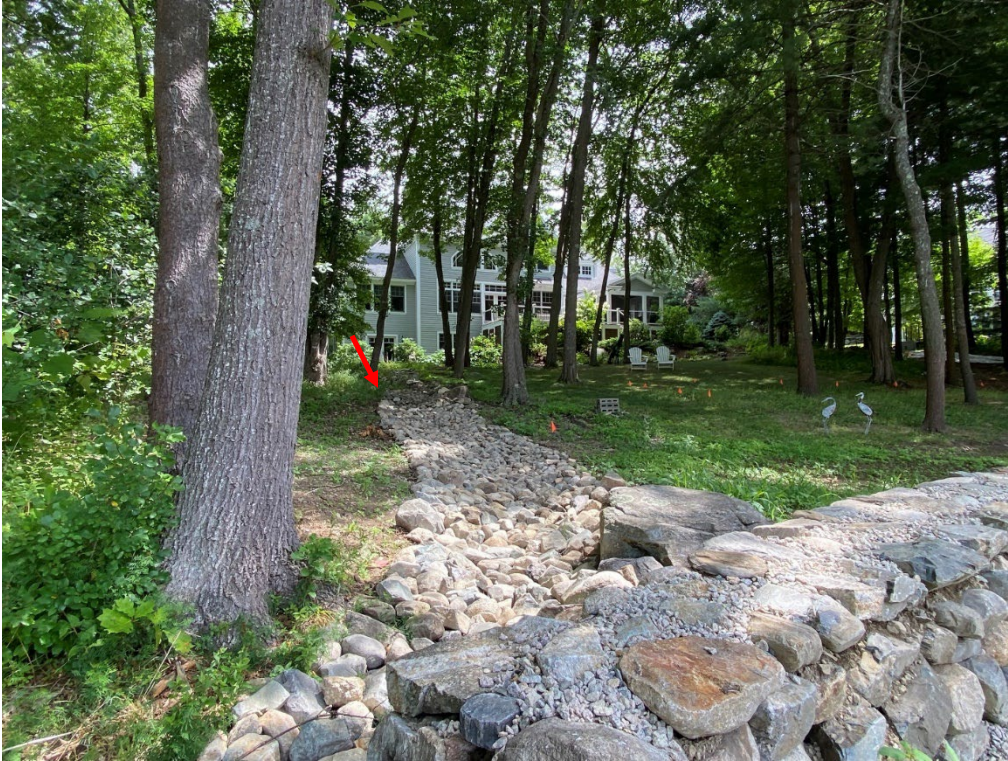
Photo 29. Overview of the newer portion of the stone swale, viewing east from below the reconstructed stone wall. Location of the top of the stone swale extension is indicated by the red arrow. (08-11-22)
