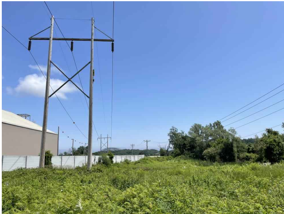
Photograph No. 30: Looking east at Structure 6 and Wetland PW-7 (PEM1/PSS1E,H) on the T13 Line ROW off Gosling Road, Portsmouth, NH.
