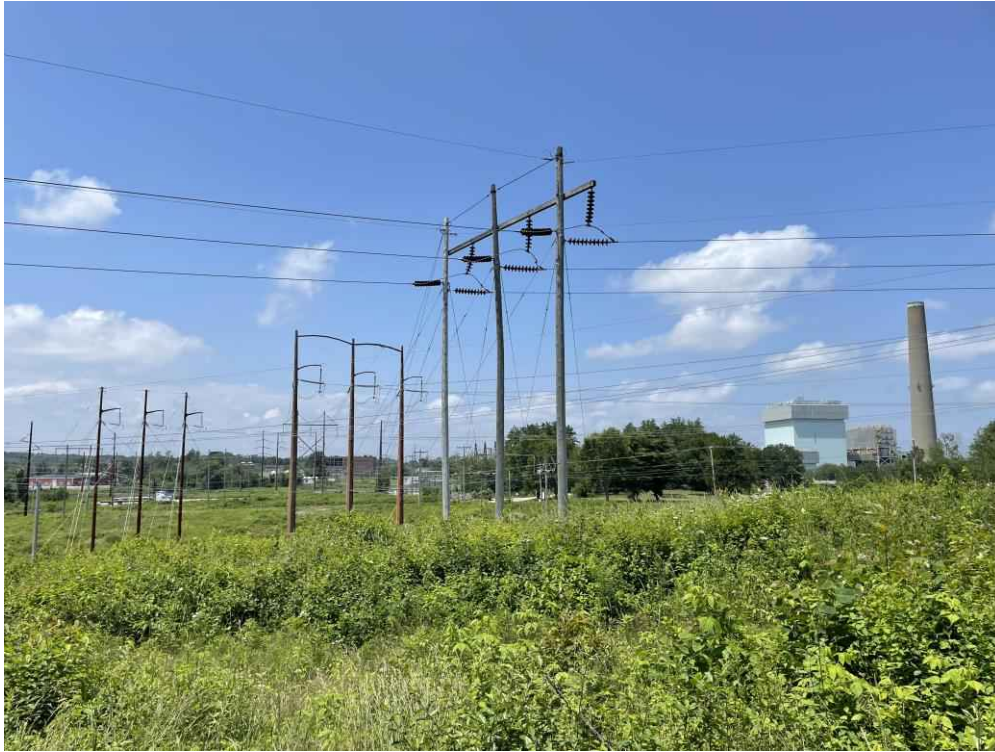
Photograph No. 23: Looking northwest near Wetland PW-3 (PEM1/PSS1E) between Structures 1 and 2 on the T13 Line ROW off Gosling Road, Portsmouth, NH.
