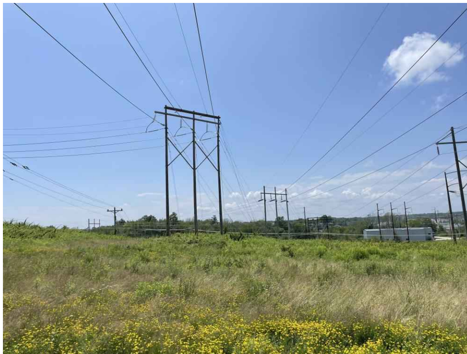
Photograph No. 24: Looking southwest at Structure 2 on the T13 Line ROW off Gosling Road, Portsmouth, NH.
