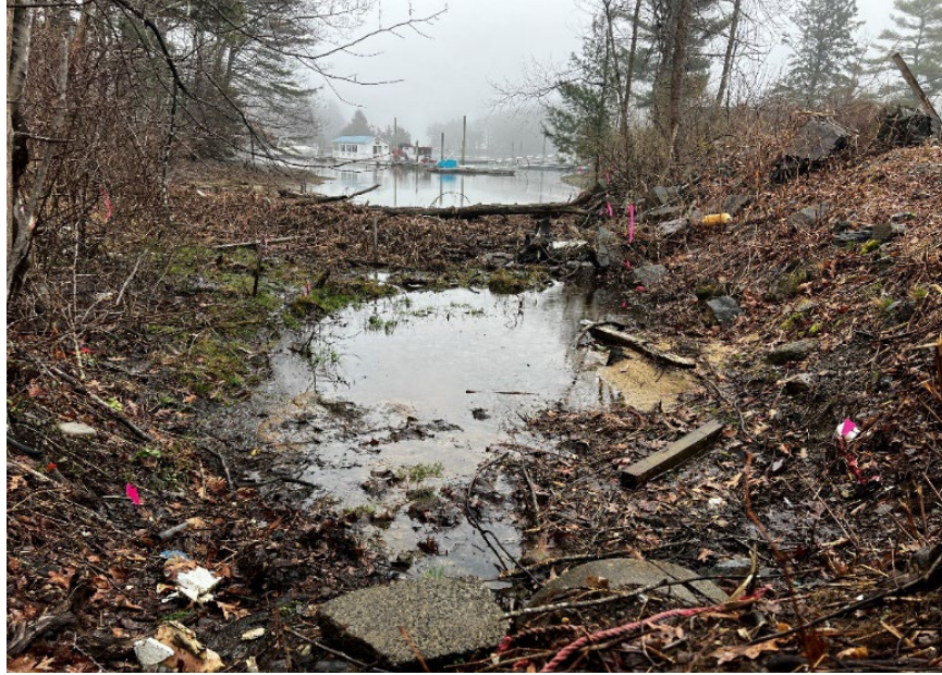
Photograph 9a: Looking east from storm drain pipe, note eroded bank along right, shows entire wetland remediation area; April 2024
