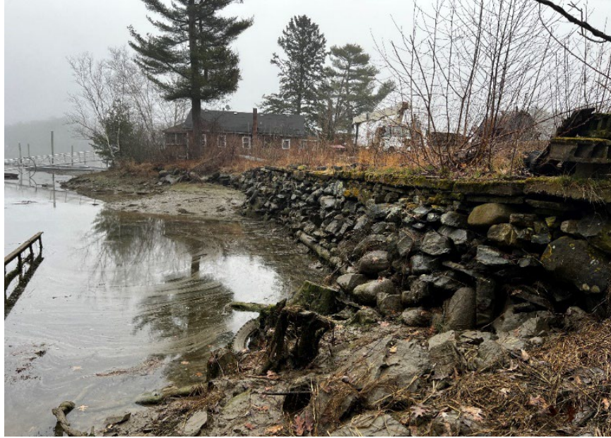
Photograph 5a: Looking south, view of cribbed stone retaining wall, from A-10 eastward (see Sheet 5); April 2024
