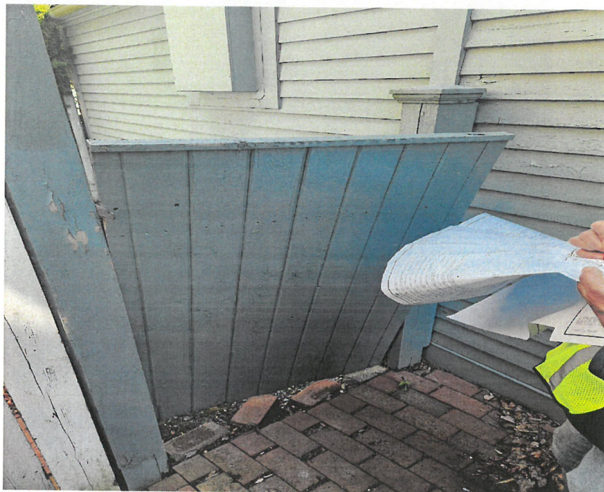
Photo #2: Looking northly at the broken gate. April 28, 2025
