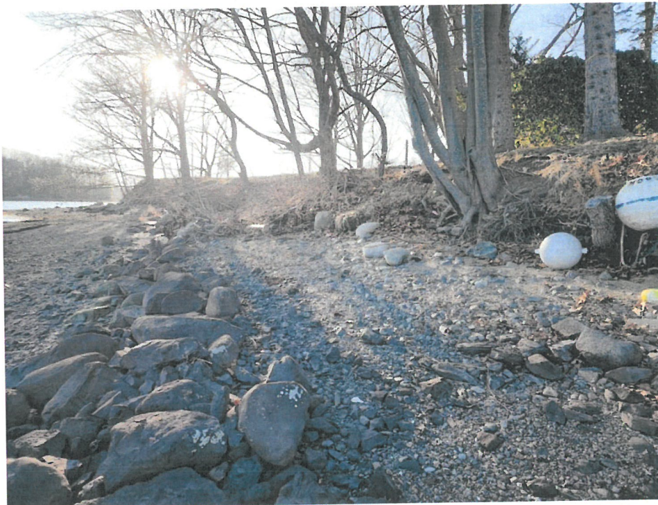
Photo #27: Looking westerly at erosion damage at shoreline interface at abutting property line. - March 1, 2024
