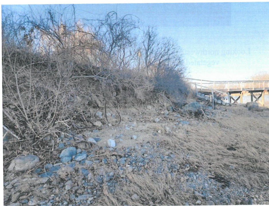
Photo #19: Looking northeasterly at existing erosion damage at shoreline and bluff. Proposed coir logs to be installed with native plantings. - March 1, 2024
