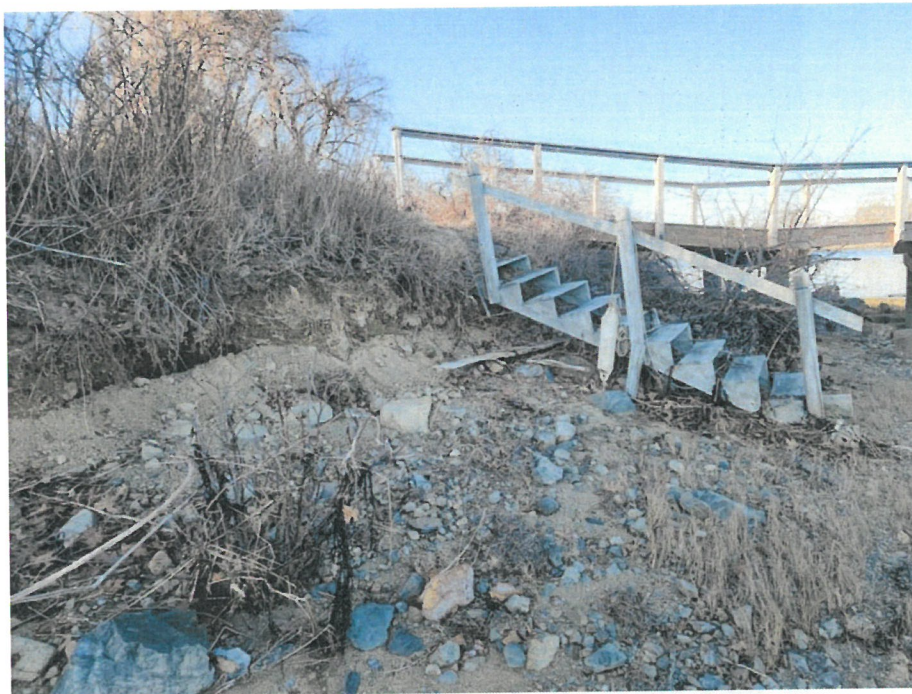
Photo #18: Looking northerly at erosion at shoreline and Piscataqua River interface. March 1, 2024
