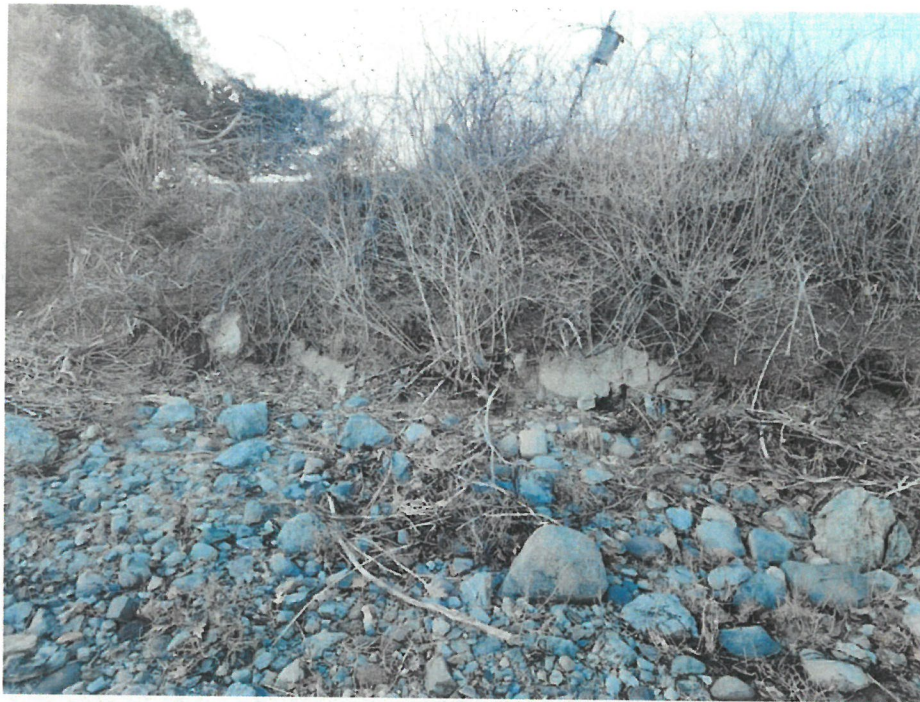
Photo #20: Looking northwesterly at severely eroded bank of the bluff from shoreline. It is proposed a living shoreline be installed in this area. March 1, 2024
