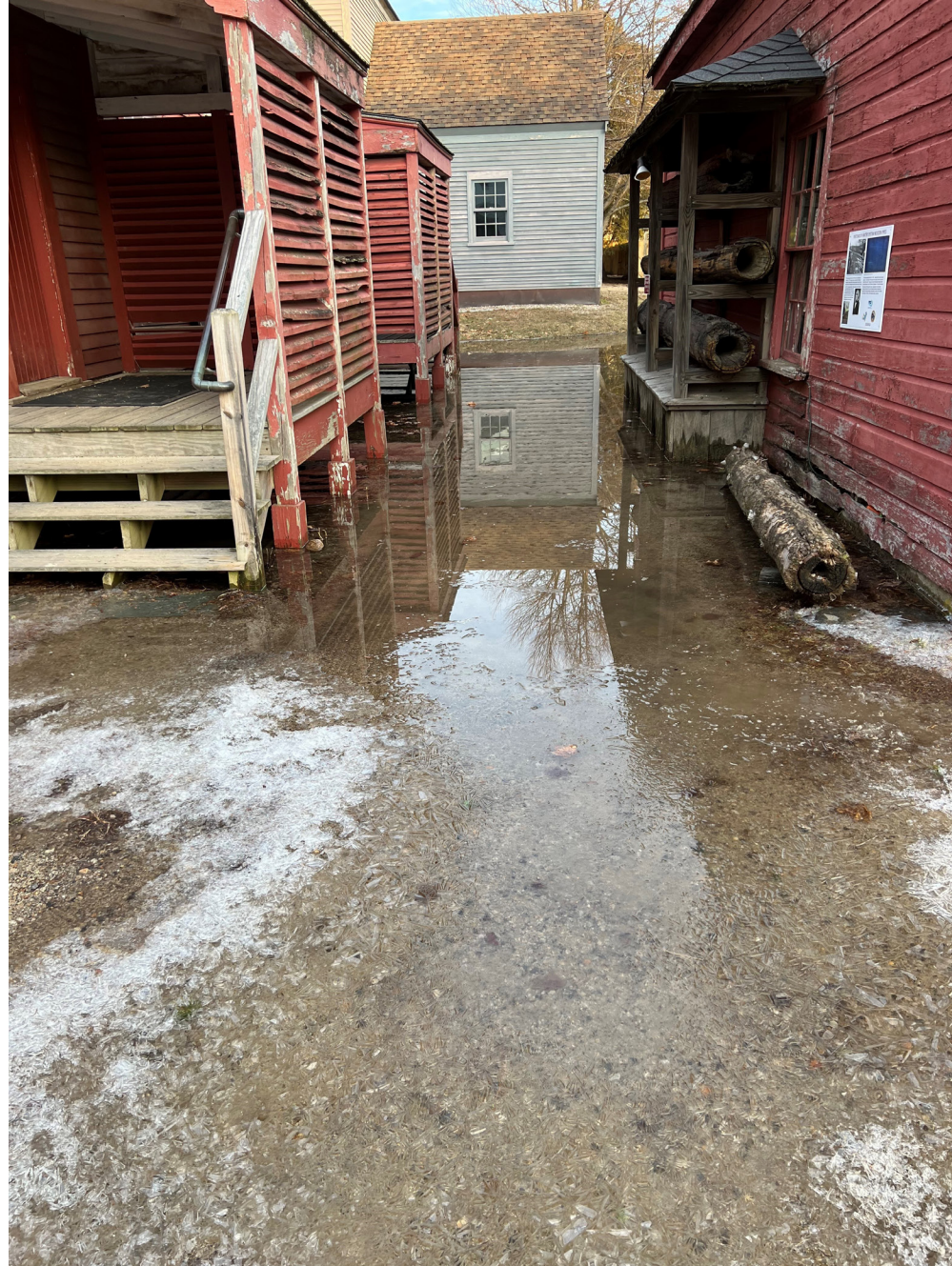
FLOODING AT PENHALLOW REAR
