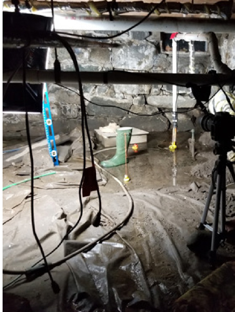
FLOODING AT PENHALLOW REAR
