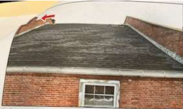
1.0 Item 21(Picture) falling parapet wall
