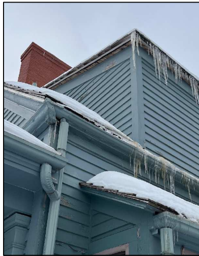
1. BACK DORMER EAVE CONDITION To be rebuilt to match front dormer
