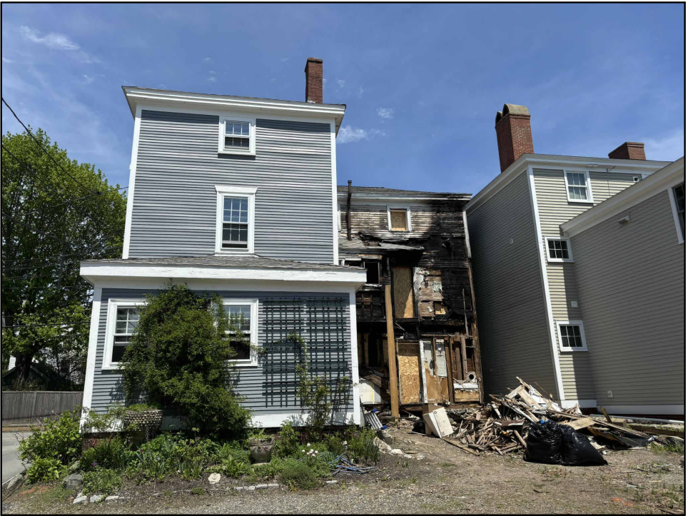
REMAINDER OF BURNED SOUTHEAST ADDITION
