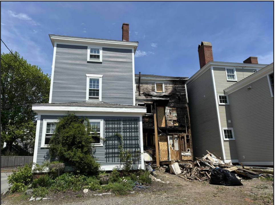
REMAINDER OF BURNED SOUTHEAST ADDITION
