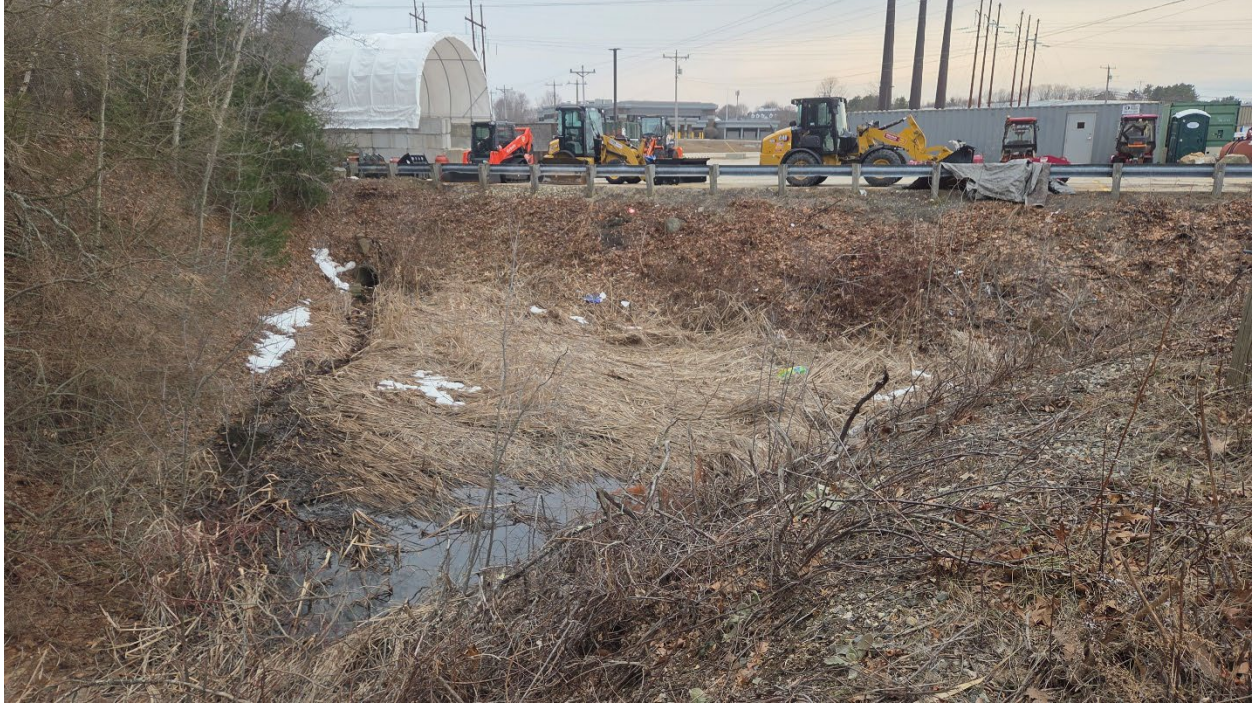
Photo 11 – Liberty Mutual – View looking west within the Stormwater Area and towards the outlet of Culvert $4 (Photo taken 3/20/2026).
