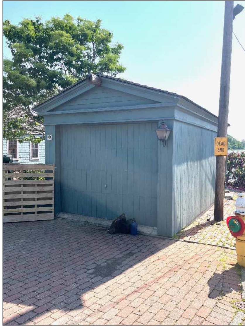
1. Garage Elevation Facing Pray Street Garage Door to be replaced. (See 2/Page 4)
