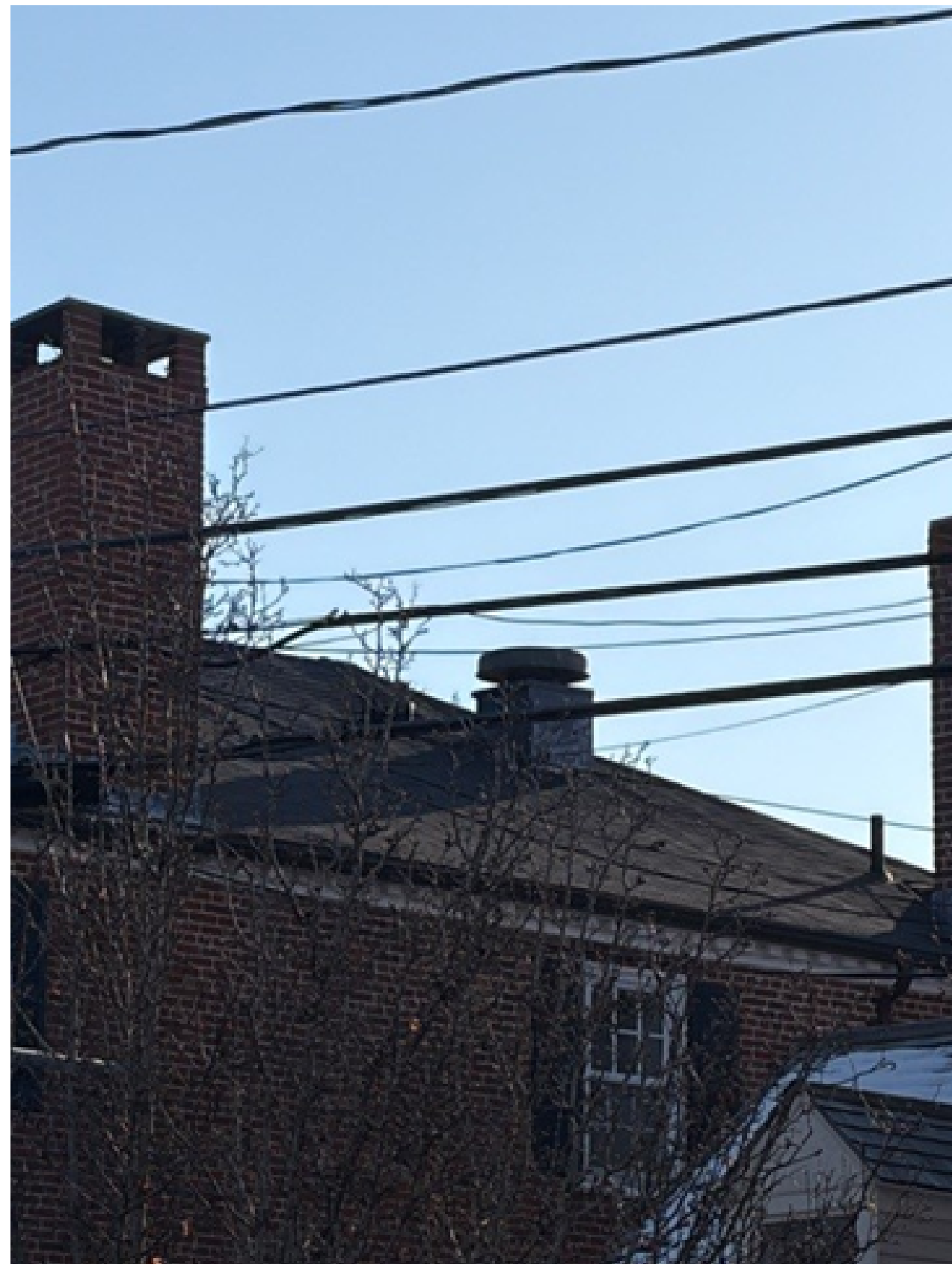
Existing Pancake Hood seen from State Street. Abandoned Duct is to the left and not clearly visible.
